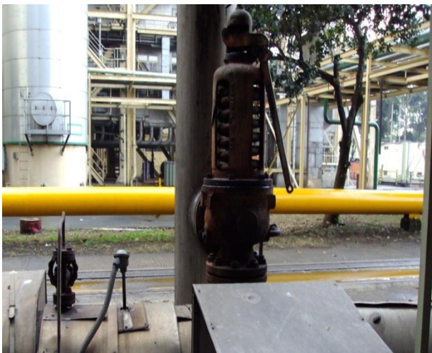
Figure 6-6: Safety valve used in APSCL
