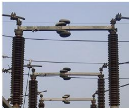
Figure 4-7: Isolator used in APSCL
