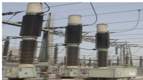
Figure 4-11: Oil circuit breaker
