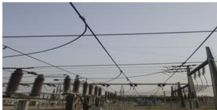
Figure 4-1: A typical bus bar of APSCL
