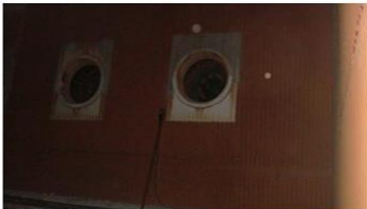
Figure 2-4: Burner room with water tube boiler
