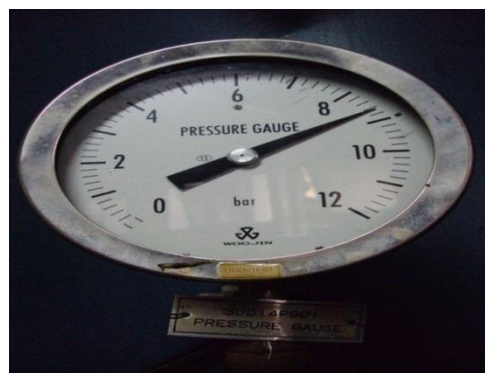
Figure 6-7: Typical pressure gauge.
