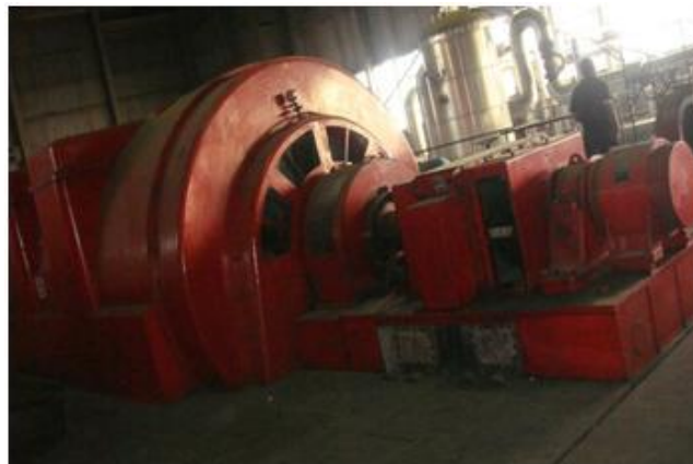
Figure 5-1: Generator in APSCL
