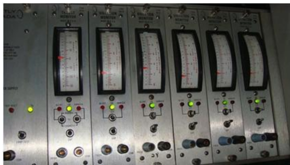
Figure 6-4: Combine cycle control unit
