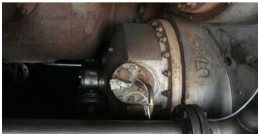
Figure 3-2: Combustion chamber in CCPP
