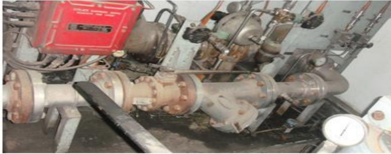
Figure 3-4: Fuel annex room in CCPP
