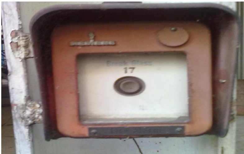
Figure 6-10: Fire alarm used in APSCCL
