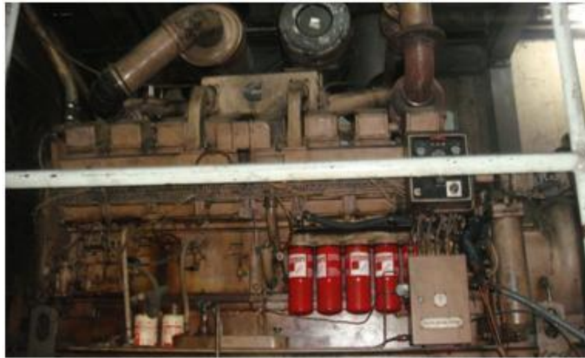
Figure 3-3: Diesel engine of CCPP
