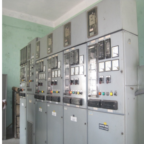
Fig4.10: Indoor type Circuit breaker
