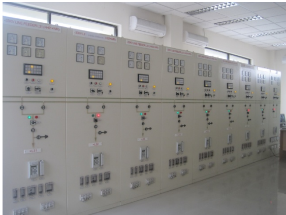
Fig4.6: X-former and line feeder panel
