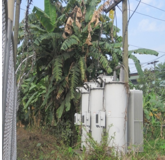
Fig4.17: LVR (line voltage regulator)
