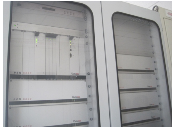
Fig4.7: Digital fault recorder
