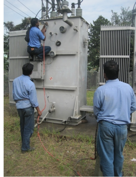
Fig5.1: checking a x-former
