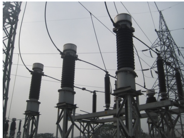
Fig-4.1: Grid Current transformer
