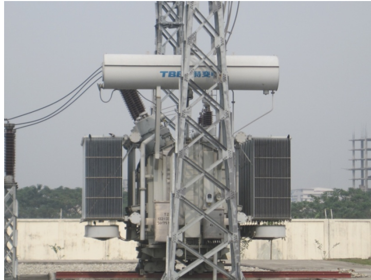
Fig-4.2: 132/33KV X-former in Grid Sub-station
