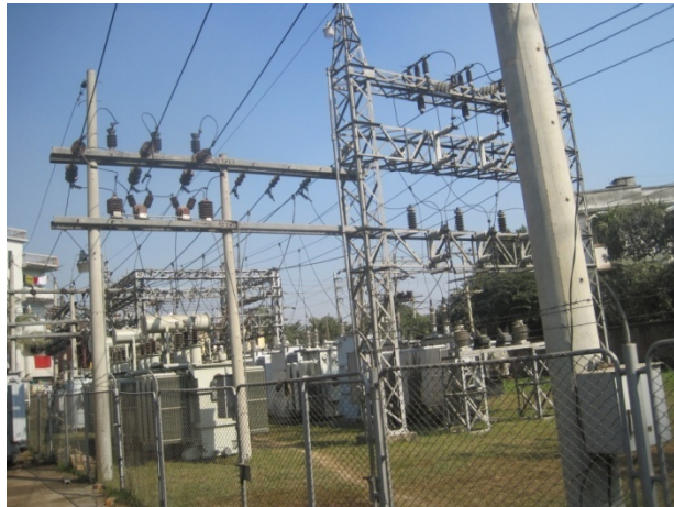
Fig4.8: Dhaka Palli Bidyut Samity-01 Power sub-station (33/11KVA)
