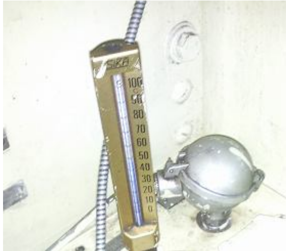
Figure 5.10: Temperature sensor & meter of turbine (Unit 3).
