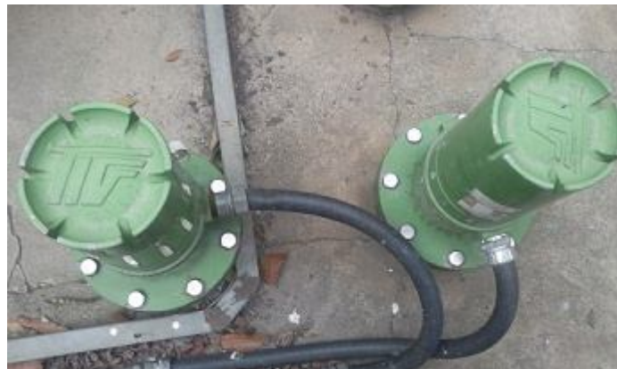
Figure 5.3: Water Level Sensor of waste water basin (Unit 3).
