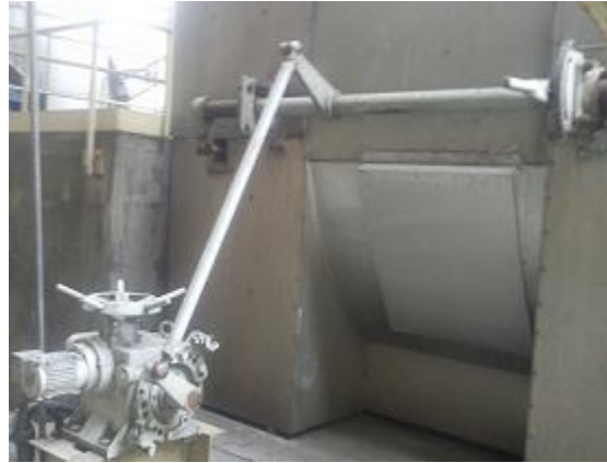
Figure 5.6: Damper of Force draft fan (Unit 4).
