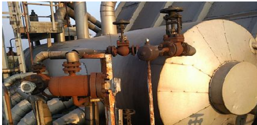
Figure 3.8: HP Boiler Drum of Waste Heat Recovery Unit.
