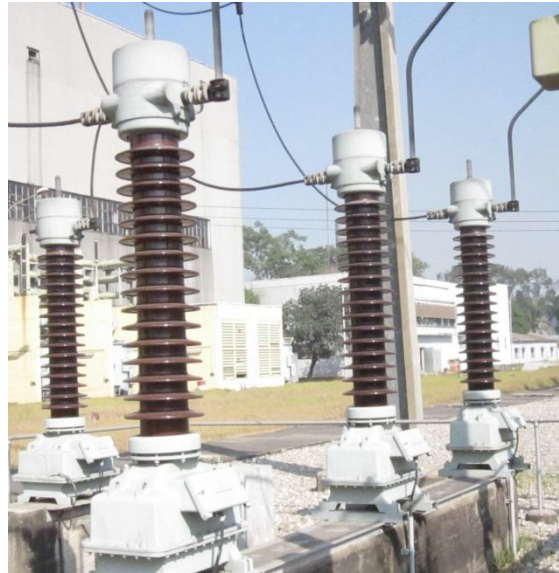
Figure 4.10: 145 kV Current Transformer in APSCCL.
