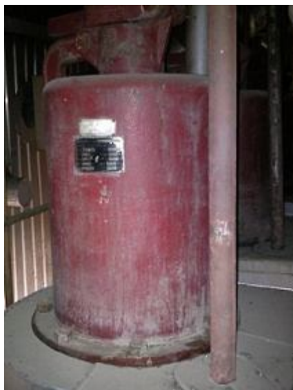
Figure 5.18: Supper heater safety valve (Unit 3 Boiler).
