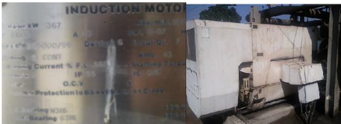
Figure 3.10: Feed Water Pump of waste heat recovery unit.
