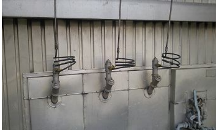
Figure 5.19: Thermostat of boiler (Unit 3, Boiler).
