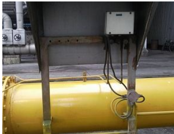
Figure 5.16: Gas flow transmitter (Unit 4).
