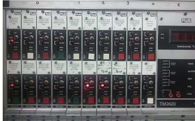
Figure 3.15: Temperature measuring panel of CCPP.
