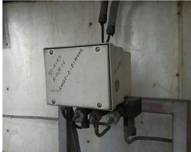
Figure 5.17: Air flow transmitter (Unit 3)
