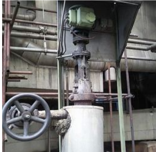
Figure 5.15: Steam pressure reducing valve (Unit 4).
