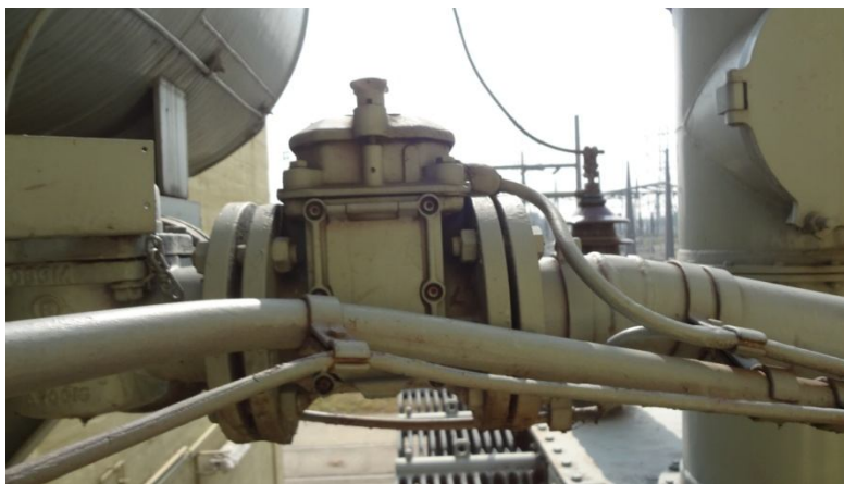
Figure 4.7 : Buchholz relay of 132 KV Transformer.
