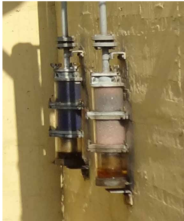
Figure 4.4 : Clear view type Silicage1 Breather of 132 KV Transformer.
