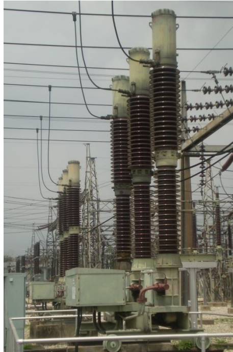
Figure 4.12: 132 KV Minimum Oil Circuit Breaker in APSC.
