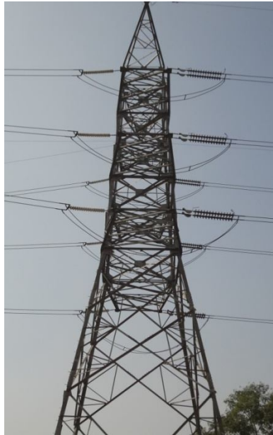
Figure 4.18: Lattice steel towers Line Supports in APSCCL.
