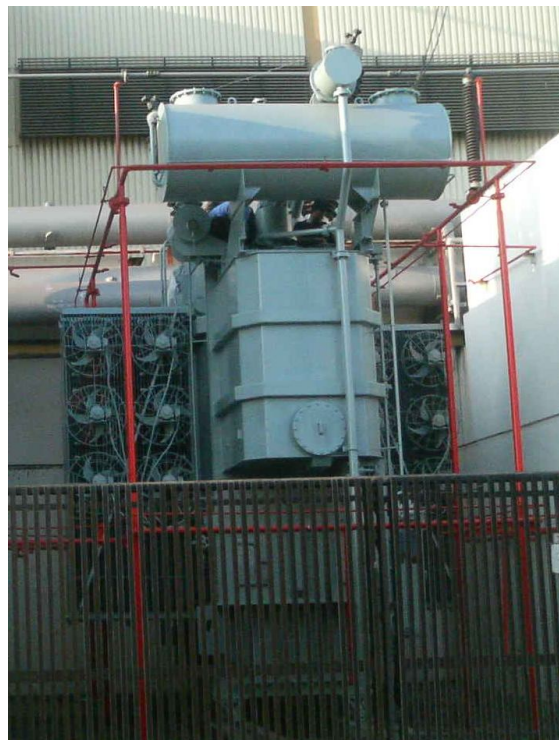
Figure 4.3: 15.75 KV/132 KV Power Transformers in APSCL.
