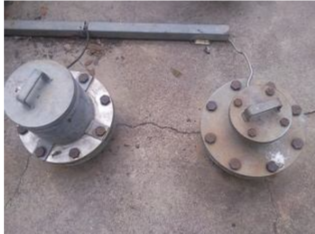
Figure 5.4: Temperature Sensor of waste water basin (Unit 3).
