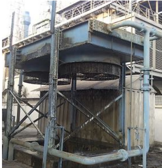
Figure 3.6: Lube Oil cooling plant
