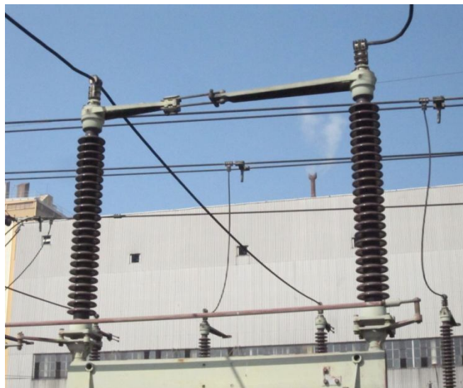
Figure 4.14 : 132 KV Isolator in APSCL.
