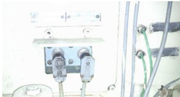
Figure 5.14: Shaft position sensor of turbine (Unit 3).
