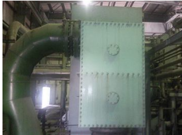
Figure 3.11: Condenser of steam turbine generator plant.
