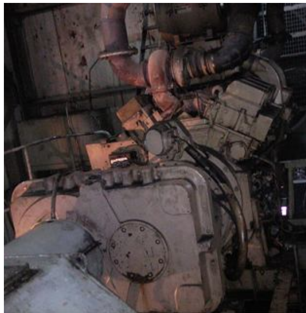
Figure 3.3: Diesel Engine of gas turbine generator section, 55.67MW.
