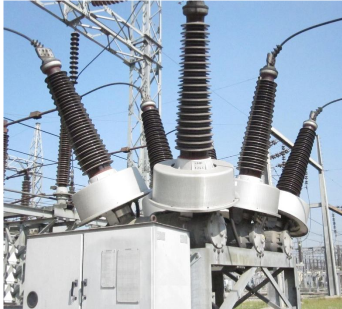
Figure 4.13: 145KV SF6 Circuit Breaker in APSCL.
