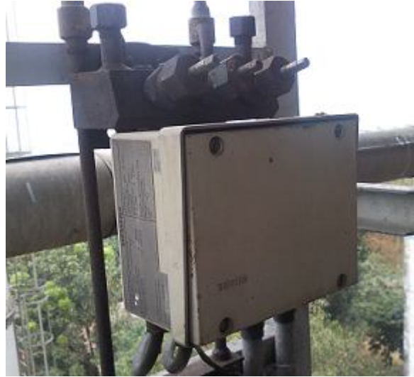
Figure 5.21: Boiler drum water level transmitter (Unit 2, Boiler).
