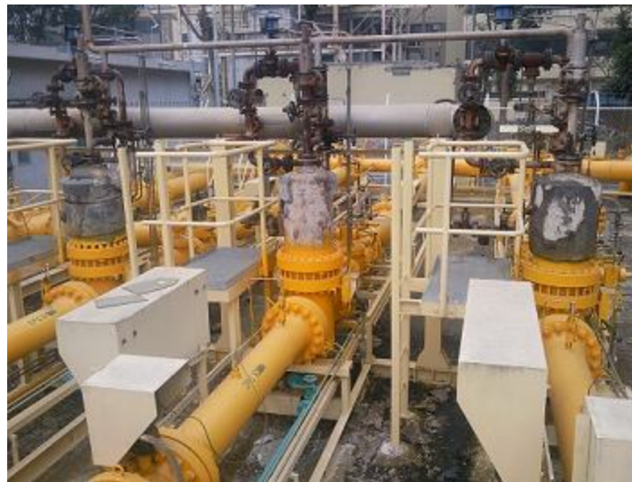
Figure 5.1: Gas Heater of gas pressure reducing plant (Unit 1, 2, 3 & 4).
