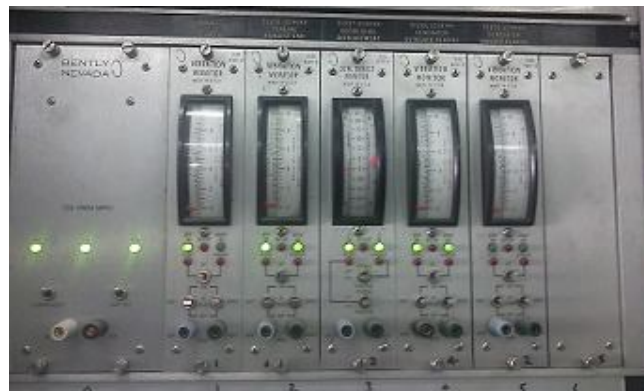
Figure 3.16: Vibration checking meter of CCPP.
