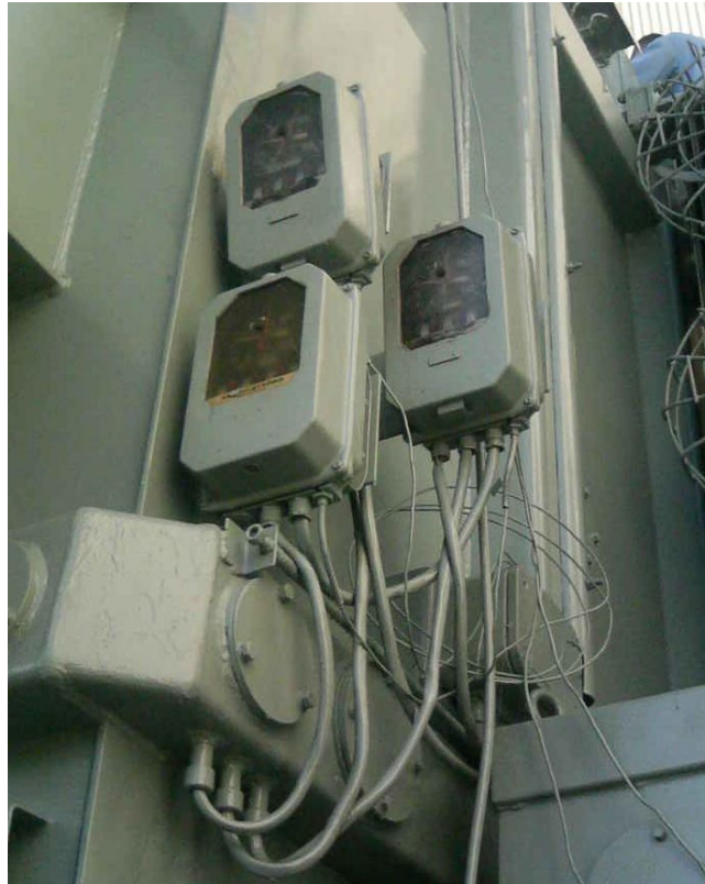
Figure 4.5 :Oil temperature and winding temperature meter of 132 KV Transformer.
