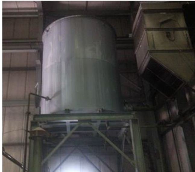
Figure 3.9: Make-Up water Tank of steam turbine generator plant.
