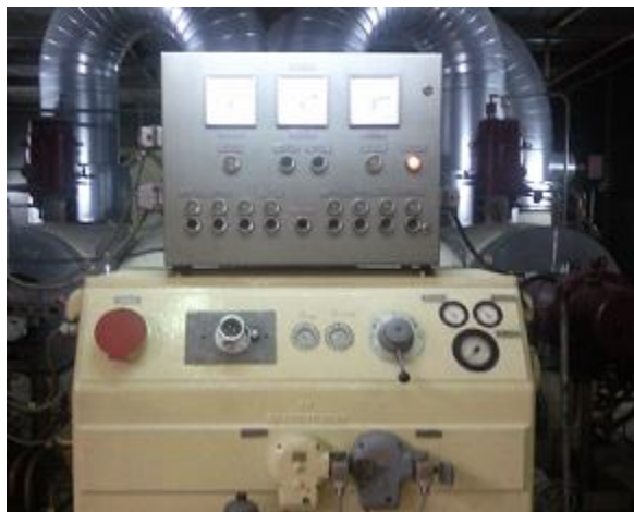
Figure 5.9: Turbine Control Panel Of Steam turbine generator plant (Unit 3).
