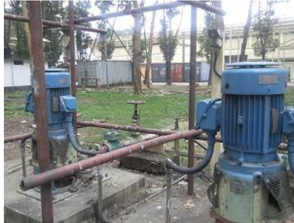
Figure 5.2: Drainage Pump of Waste water basin (Unit 3).
