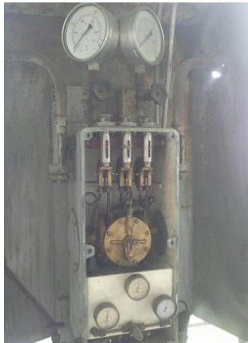
Figure 5.22: Boiler drum pressure meter ( Unit 2, Boiler).
