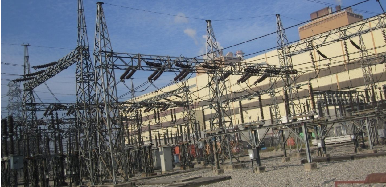
Figure 4.2: 230 KV Substation of APSCCL.
