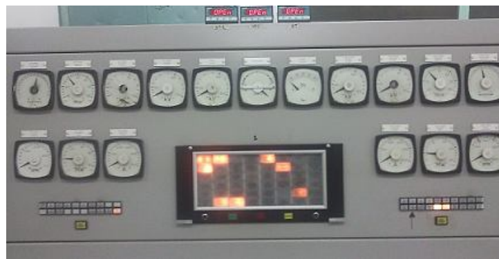
Figure 3.14: Meter Panel of CCPP.
