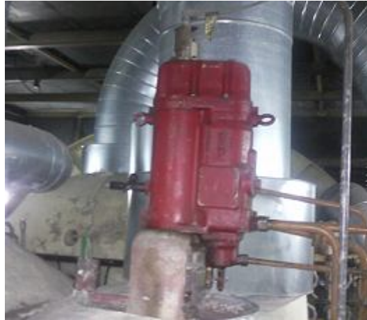
Figure 5.13: Regulating valve of turbine (Unit 3).
