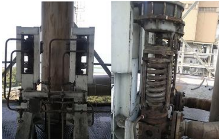
Figure 5.23: Boiler drum safety valve (Unit 2, Boiler).
