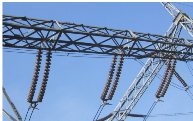
Figure 4.17: Suspension Type Insulator in 230KV substation.
