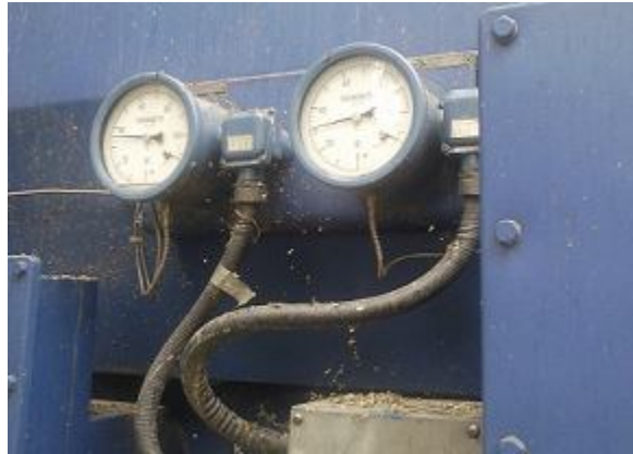
Figure 5.8: temperature sensor & meter of FD fan (Unit 4).
