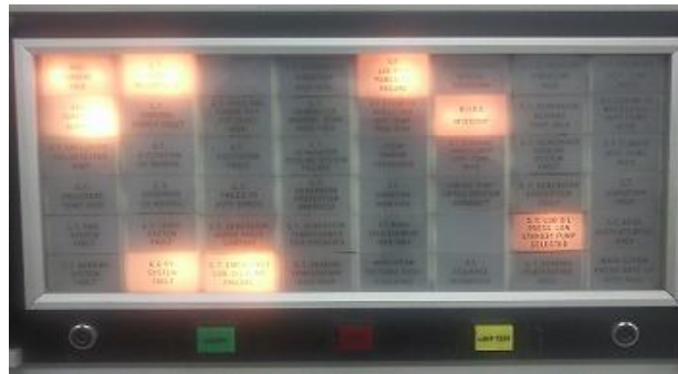
Figure 3.13: Fault Checking Interface of CCPP.
