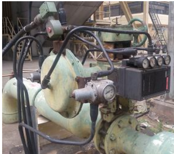
Figure 5.5: Temperature Control Actuator valve of waste water basin (Unit 3).
