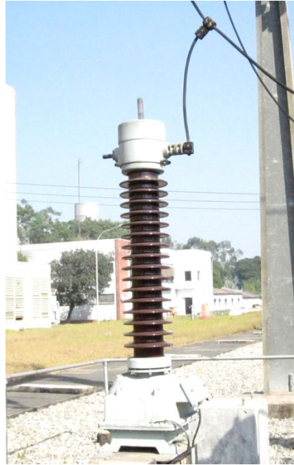
Figure 4.11: 132 kV Potential Transformer in APSCL.
