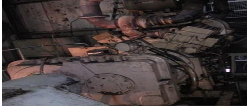
Figure 21: Diesel engine of gas turbine generator section.
