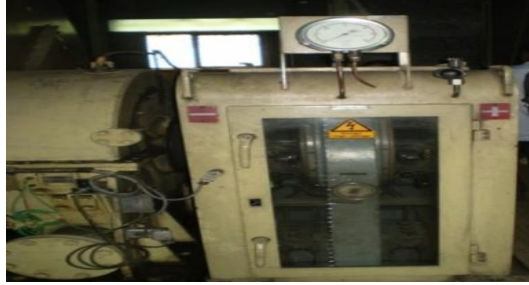
Figure 2: Static exciter used in unit 3, 4, and 5 of steam power plant of APSCL.
