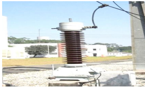
Figure 28: Potential transformer (PT).
