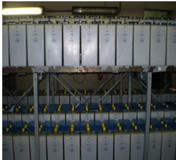
Figure 10: Battery arrangement of back-up system.
