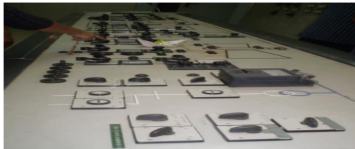
Figure 7: Control room of unit 1 and 2.
