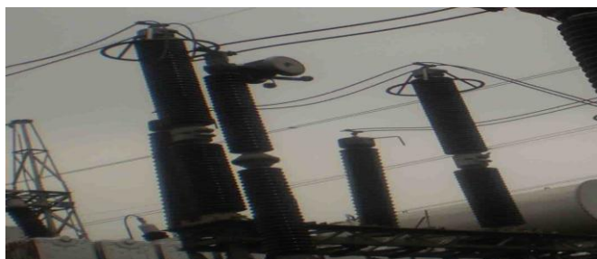
Figure 31: Zinc oxide lightning arrester.
