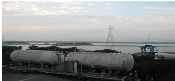
Figure 24: Feed water tank.
