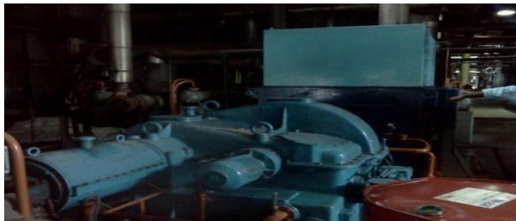
Figure 25: Feed water pump.
