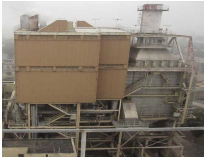
Figure 23: Generator unit 3 boiler.
