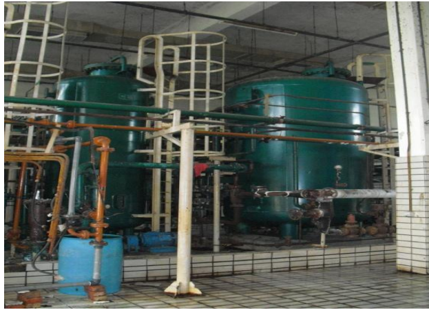
Figure 35: Demineralization filter tanks.
