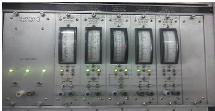
Figure 19: Vibration checking meter of CCPP control unit.
