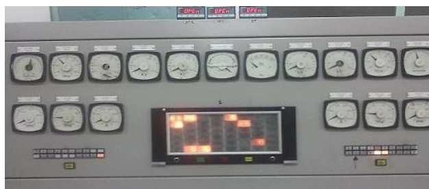
Figure 17: Meter panel of CCPP control unit.
