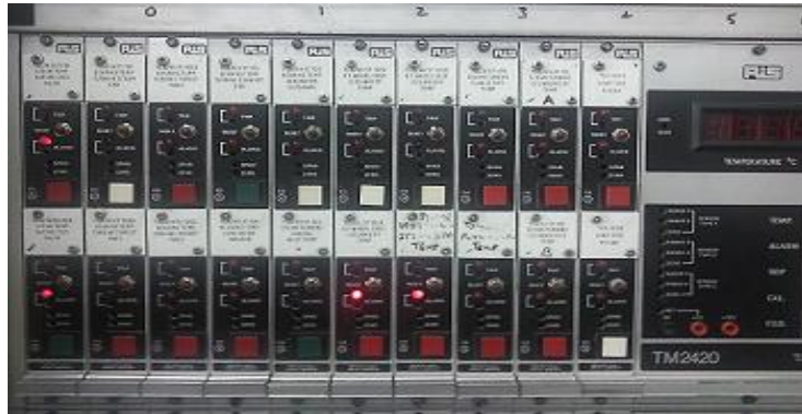
Figure 18: Temperature measuring panel of CCPP control unit.
