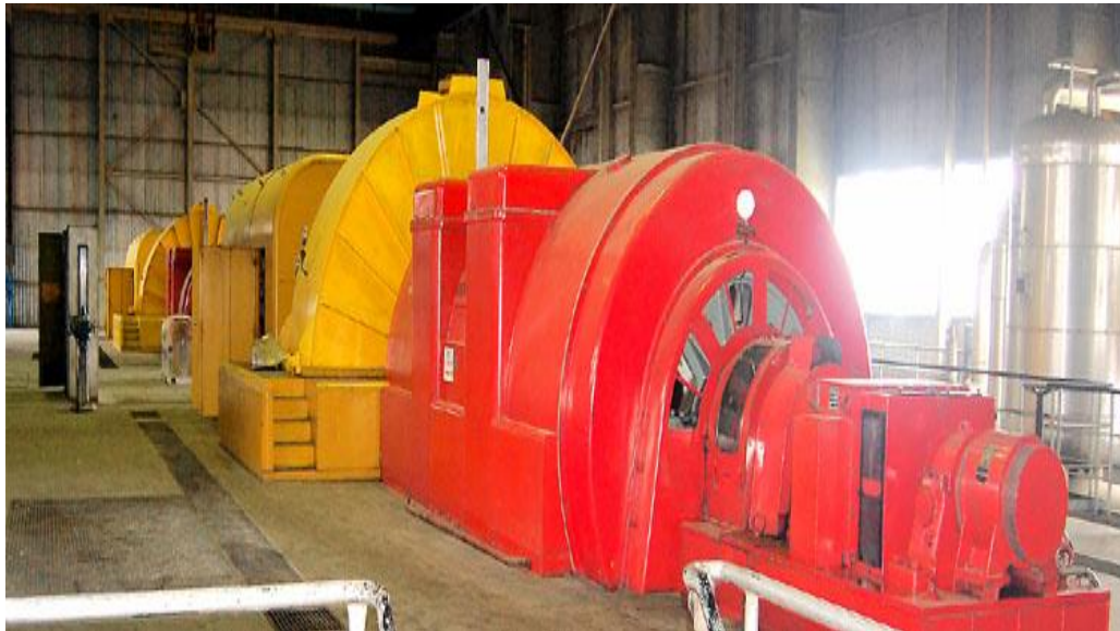
Figure 1: AC generator of ST-2.
