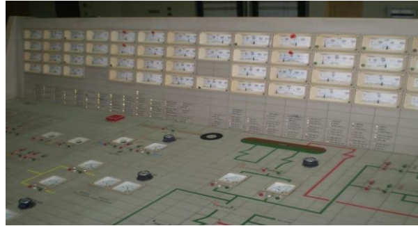
Figure 8: Control room of unit 3 and 4.
