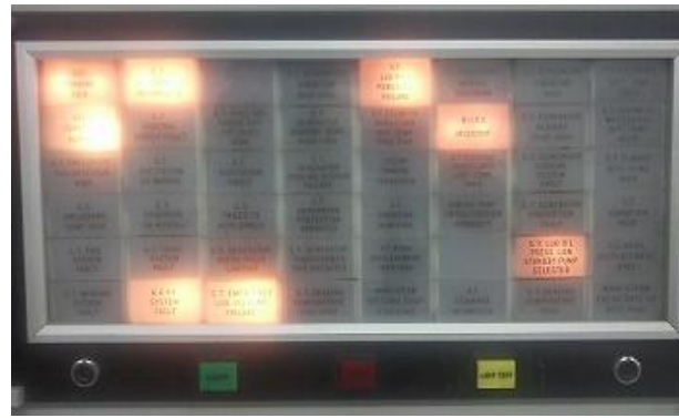
Figure 16: Fault checking interface of control unit.
