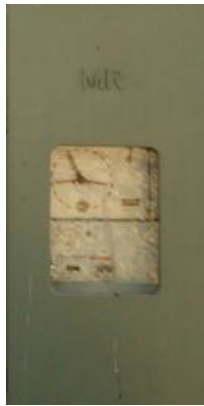
Figure 4.4: Tap changer module at DBPAL
