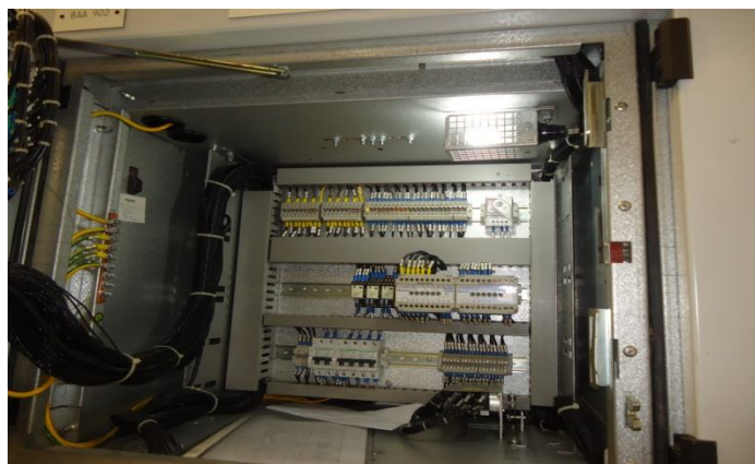
Figure 2.18: Station transformer panel
