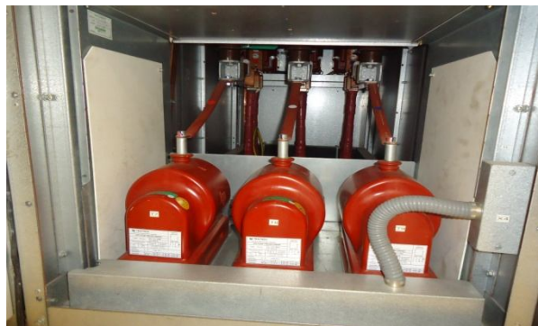
Figure 2.16: Incoming from generator panel
