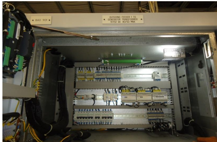
Figure 2.19: Outgoing feeder to generator panel
