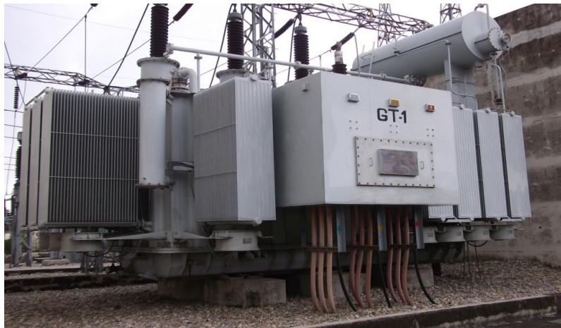
Figure 2.4: 132/33 KV Power transformer (GT1) at Uttara grid-substation .
