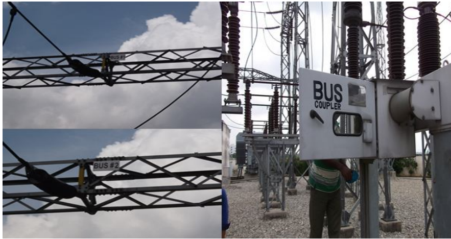
Figure 2.20: 132 KV bus bars and bus coupler at Uttara grid-substation.
