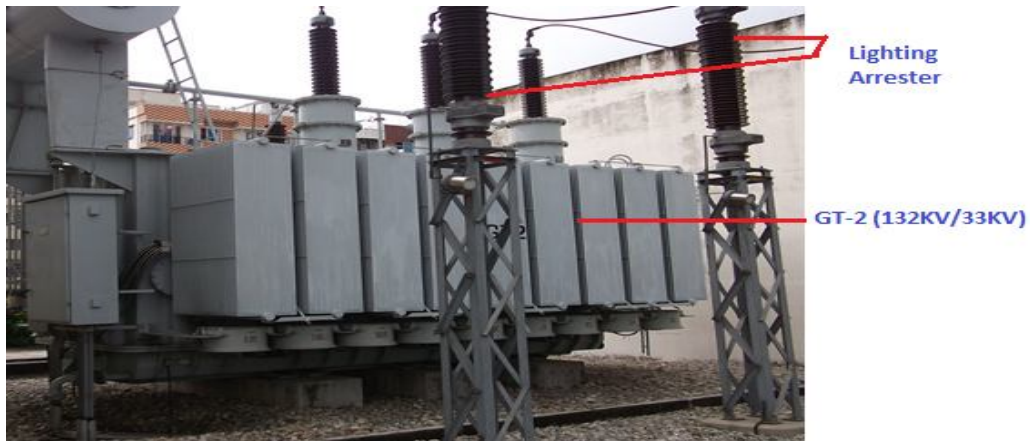
Figure 2.17: Lightning Arrester and GT-2 at Uttara grid-substation.
