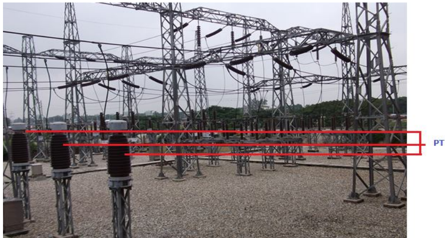
Figure 2.15: Potential transformer at Uttara grid-substation.
