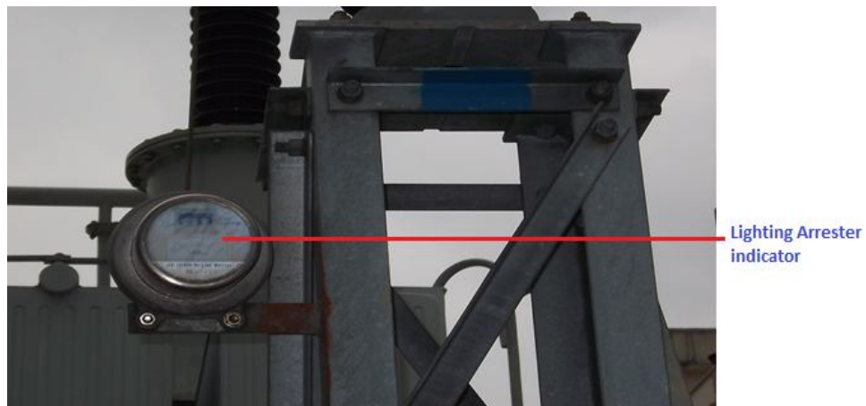
Figure 2.18: Lightning arrester indicator at Uttara grid-substation.
