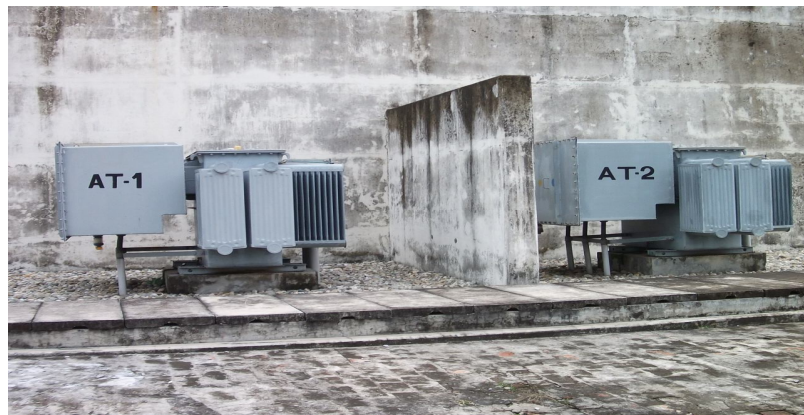
Figure 2.13: Auxiliary transformer at Uttara grid-substation.
