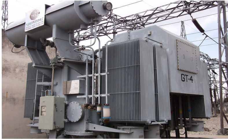
Figure 2.5: 33/11KV power transformer (GT4) at Uttara grid-substation.
