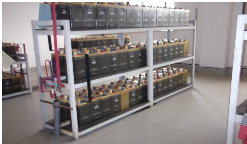
Figure 2.21: Battery back up system of 132/33/11KV Uttara grid-substation.
