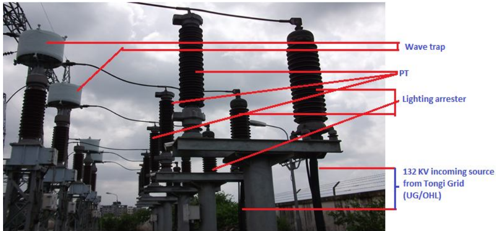
Figure 2.2: 132KV incoming source from Tongi grid, wave trap, PT and L.A.
