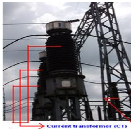
Figure 2.16: Current transformer at Uttara grid-substation.
