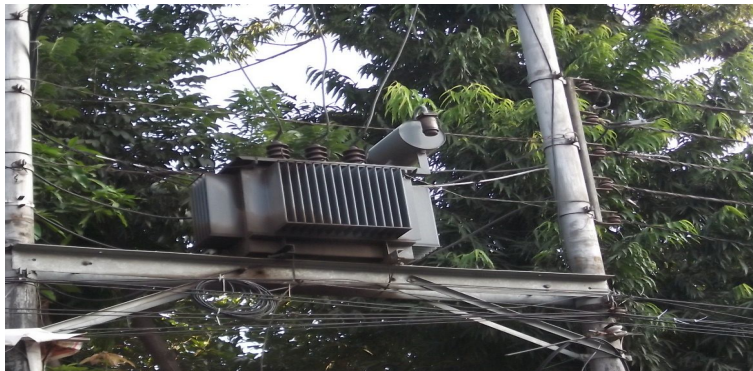
Figure 3.4: The 11/415KV distribution transformer [10].
