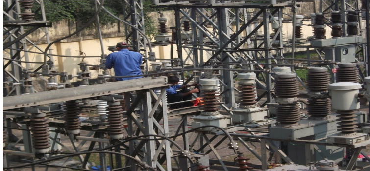
Figure 3.2: Maintenance of Kafrul (Mirpur) 33/11 KV substation.
