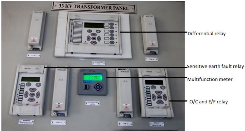
Figure 3.8: The digital relay protection on 33KV transformer panel.
