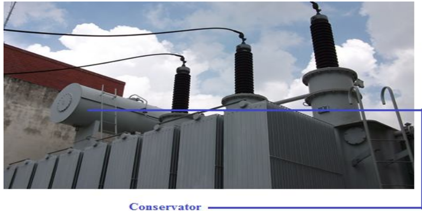
Figure 2.8: Conservator tank at Uttara grid-substation.
