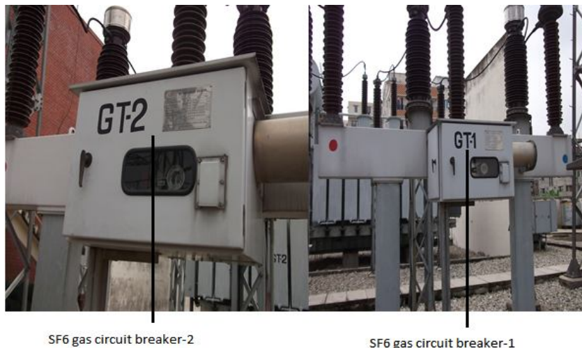
Figure 2.14: SF6 gas circuit breaker at Uttara grid-substation.
