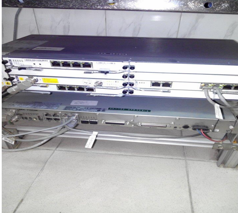
Fig01: IDU in a BTS room.
