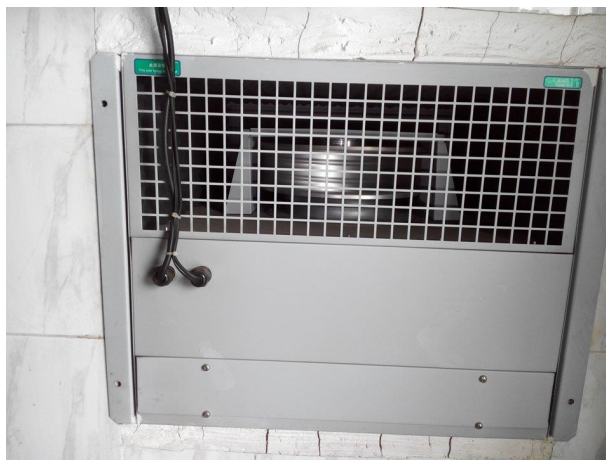
Fig07: DVS at BTS room
