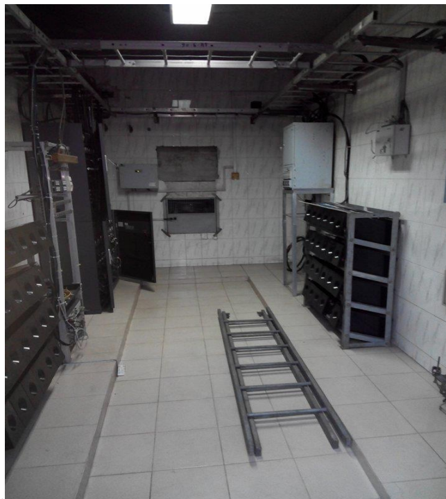
Fig23: Indoor BTS room
