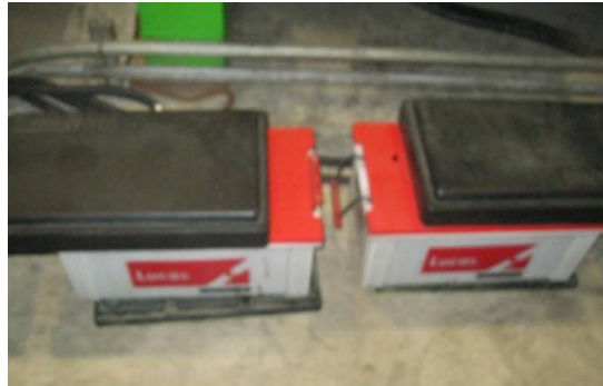
Figure 2.8: The DC storage batteries inside the engine room.
