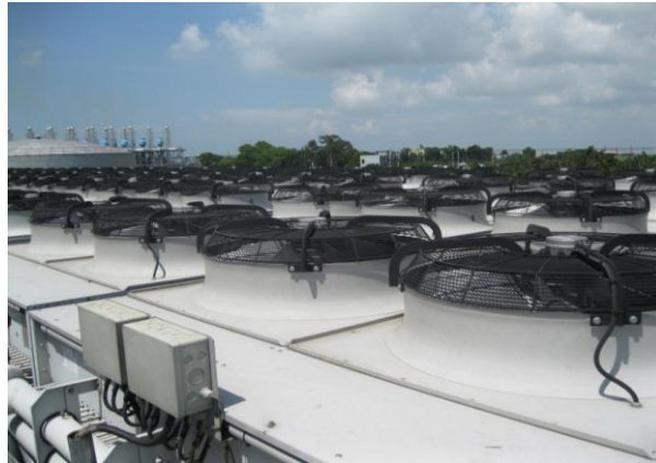
Figure 2.6: Fans in water cooling system of gas engine power plant at APSCL.
