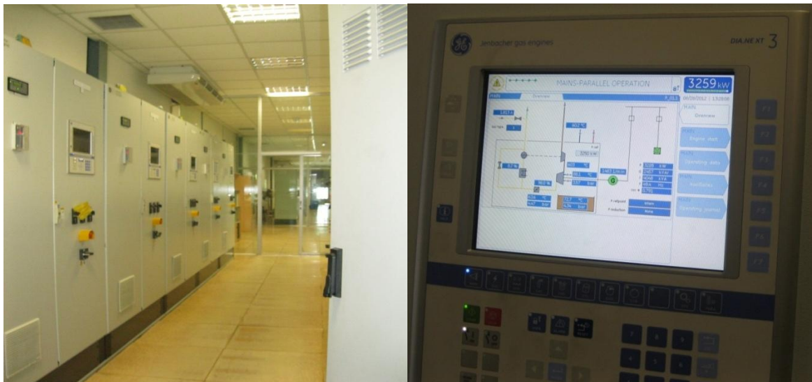
Figure 2.1: Control room (left side) and a control panel (right side) of gas engines.
