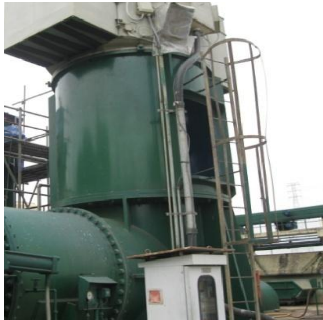
Figure 5.1: Water pump of APSCL to collect river water.
