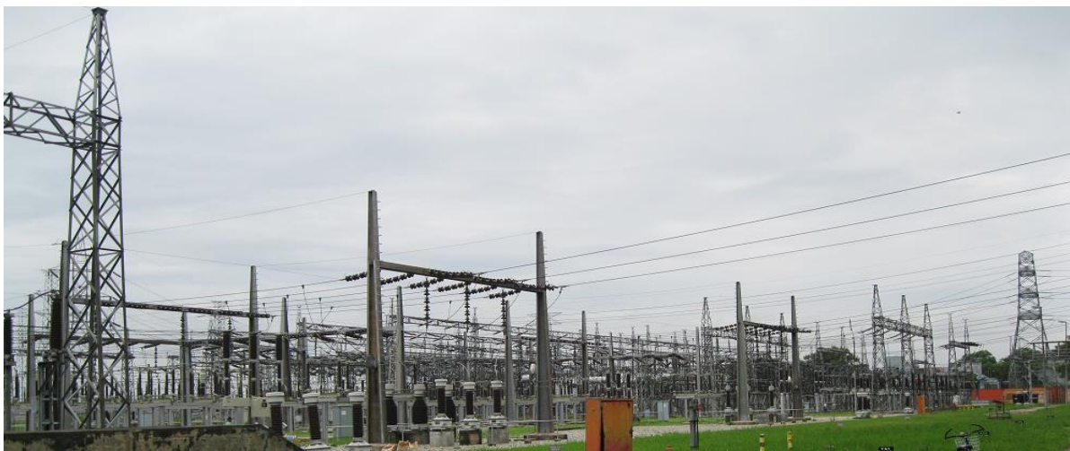
Figure 3.1: Substation of APSCL.
