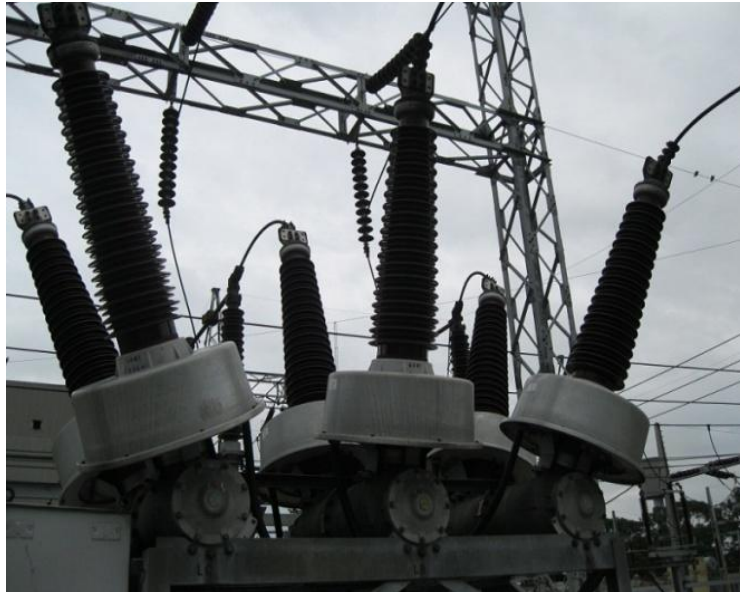
Figure 3.3: SF6 circuit breaker of APSCL switchyard.
