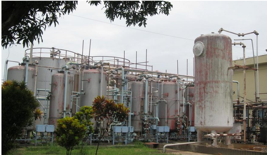
Figure 5.2: Water treatment plant of the APSCL.
