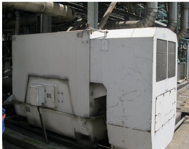
Figure 4.3: Boiler feed pump of steam turbine unit.
