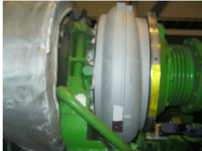
Figure 2.4: The turbo-charger inside the engine room.
