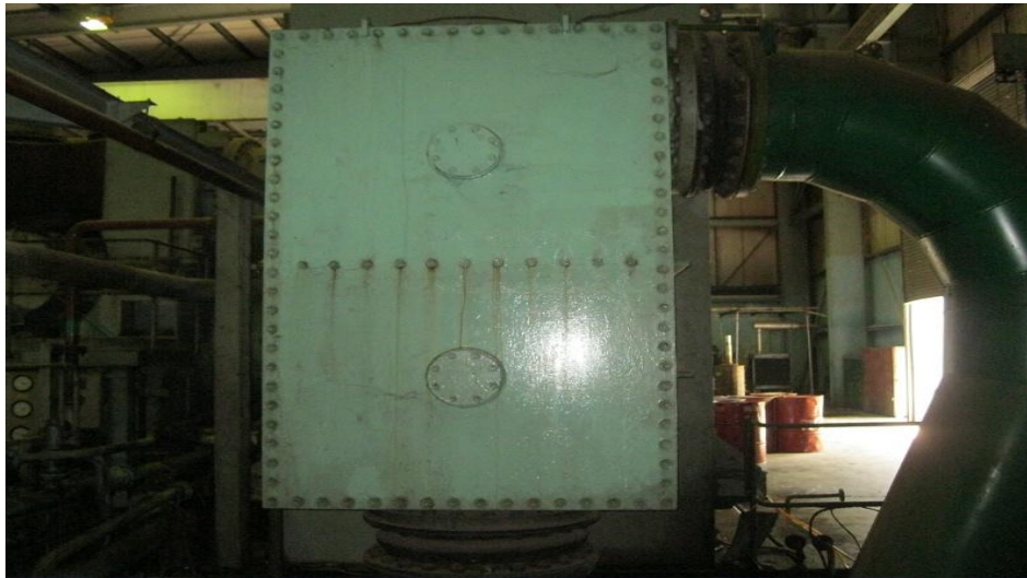
Figure 4.4: The condenser of the steam turbine unit.
