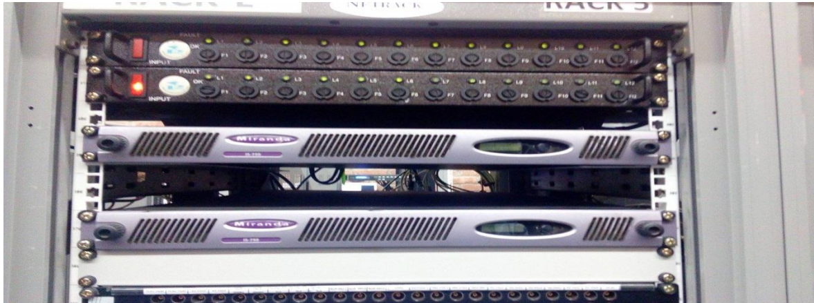
Fig: 4.10 Miranda server of ITV
