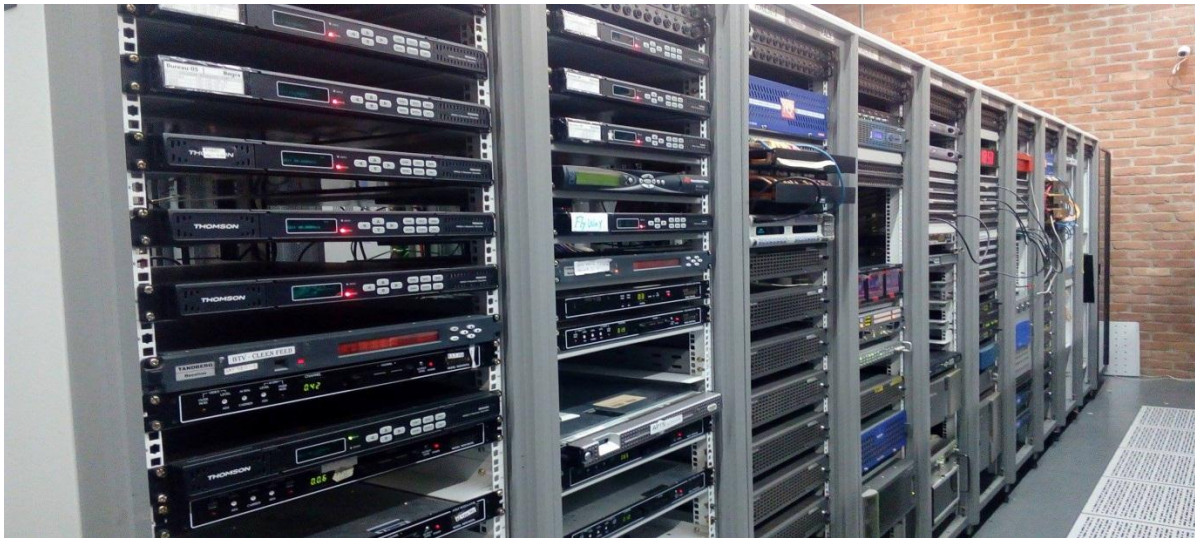
Fig 4.1: The rack in CAR of ITV
