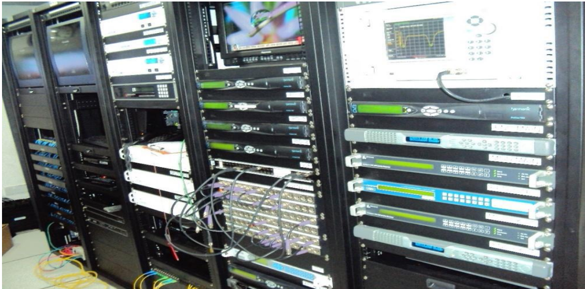
Fig 4.2: The rack in Earth Station of ITV
