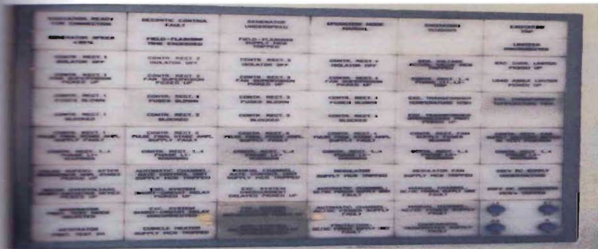
Figure 16: generator control system for fault analysis board
