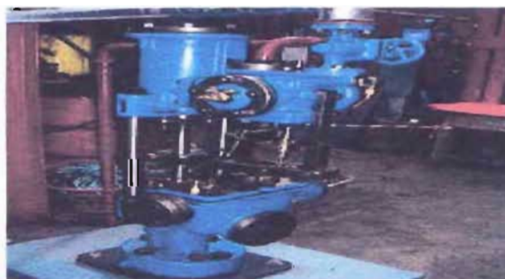
Figure 25: feed water pump
