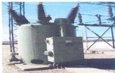
Figure 52: Bulk Oil Circuit Breaker
