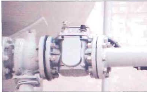
Figure 56: Buchholz relay connection
