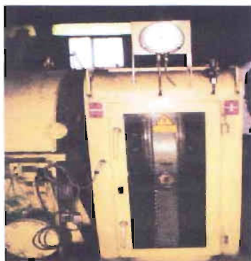
Figure 2.8: Static Exciter used in unit-3, 4, 5 of steam power plant of APSCCL
