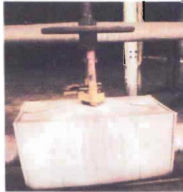
Figure 2.32: Manual valve used in combined cycle power plant of APSCL
