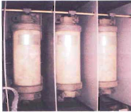
Figure 3.13: Internal part of vacuum circuit breaker
