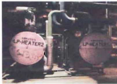
Figure 2.21: LP heater of steam power plant of APSCL
