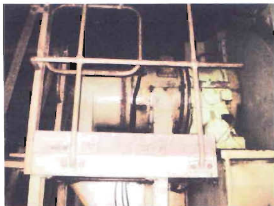
Figure 2.7 : Brushless Thyristor Excitator used in the combined cycle power plant of APSCCL
