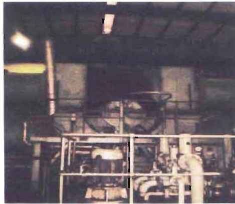
Figure 2.28: Gas turbine of APSCL
