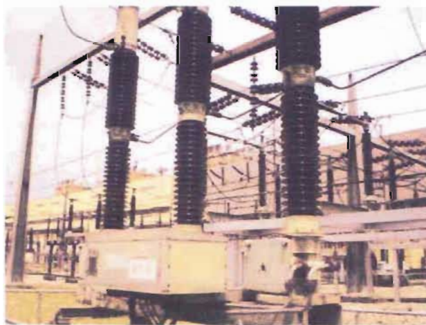
Figure 4.6: Oil Circuit Breaker at APSCL
