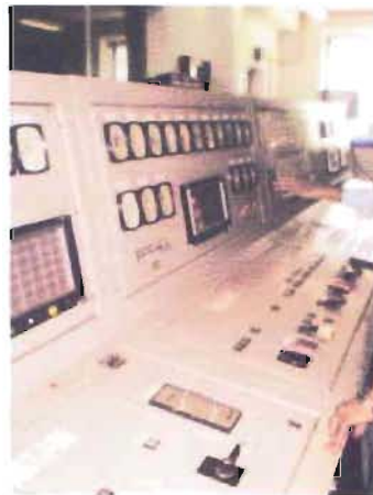
Figure 3.24: Control Room of combine cycle
