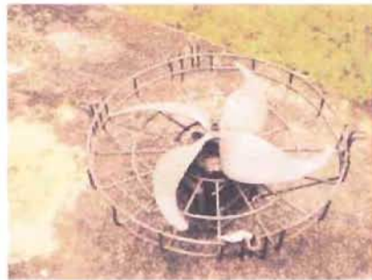
Figure 4.19: Transformer cooling fan
