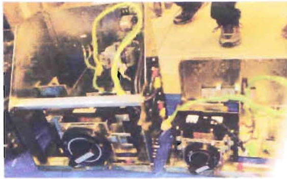
Figure 3.11: molded cage circuit breaker
