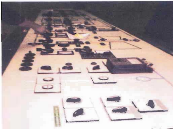
Figure 3.21: Control Room of unit 1&2
