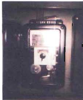
Figure 3.5: stator earth fault relay
