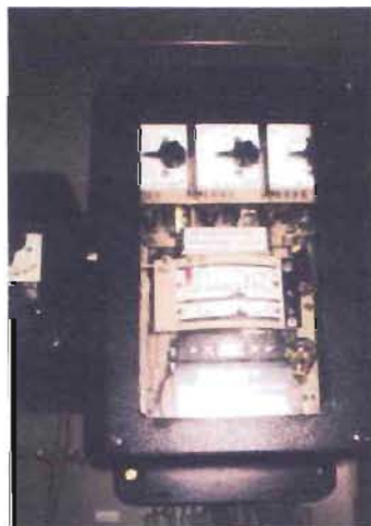
Figure 3.9: Picture of over current relay used in APSCIL.
