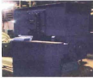
Figure 3.19: Cooling water pump
