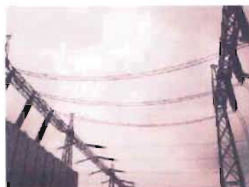
Figure 4.3: Bus Bar in APSC L
