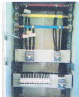
Figure 6.2: Inside of LT Switchgear
