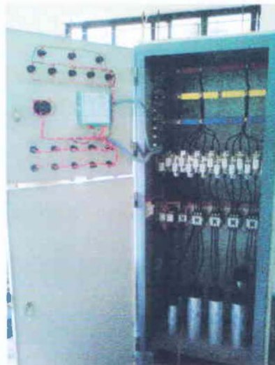
Figure 6.7: Inside of PFI plant
