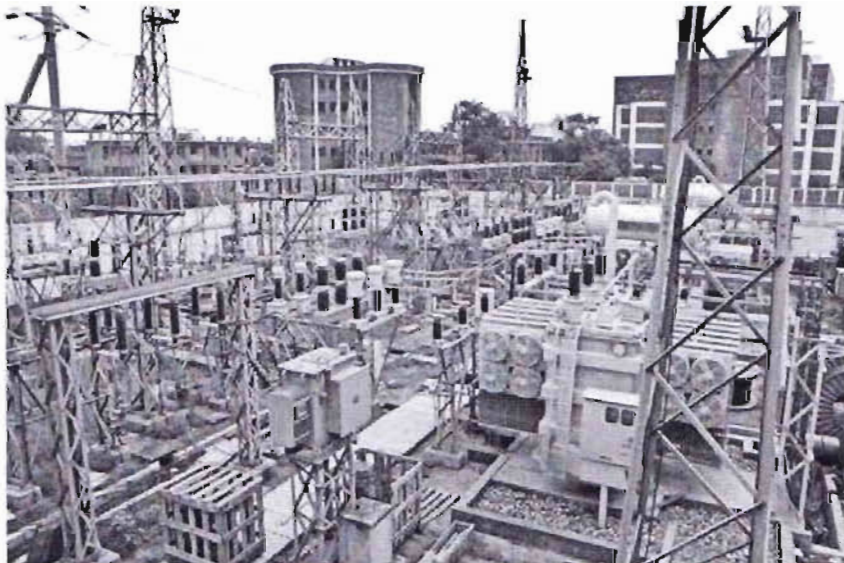
Figure 2.3.1: Kafrul substation (33 KV/11 KV).
