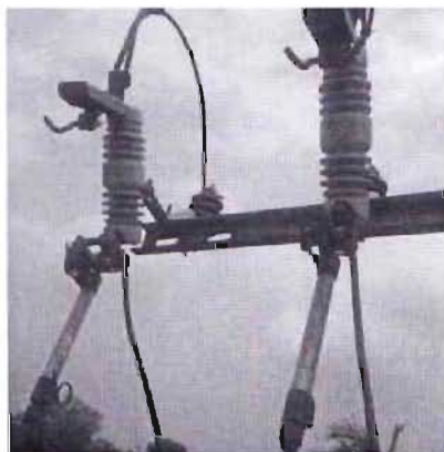
Figure 3.4.4: Transformer drop off fuse.
