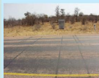
Typical installation of inductive loops.
