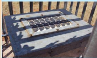
Automatic counting station secured and operated by solar power.
