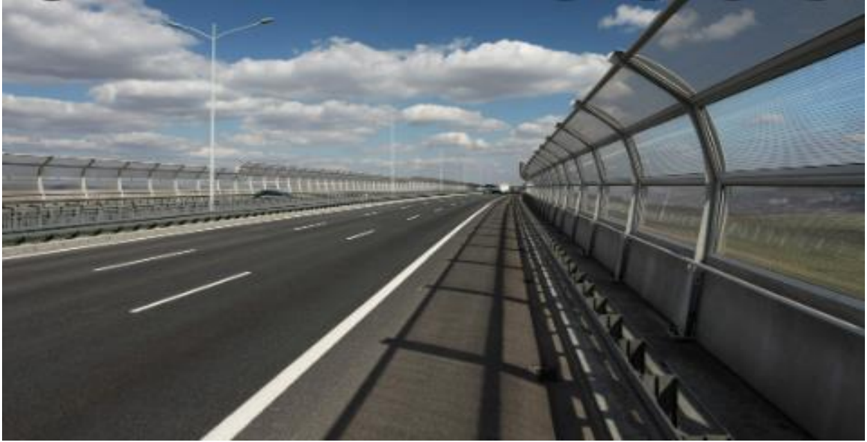
Figure 8.6 Noise barrier in highway
