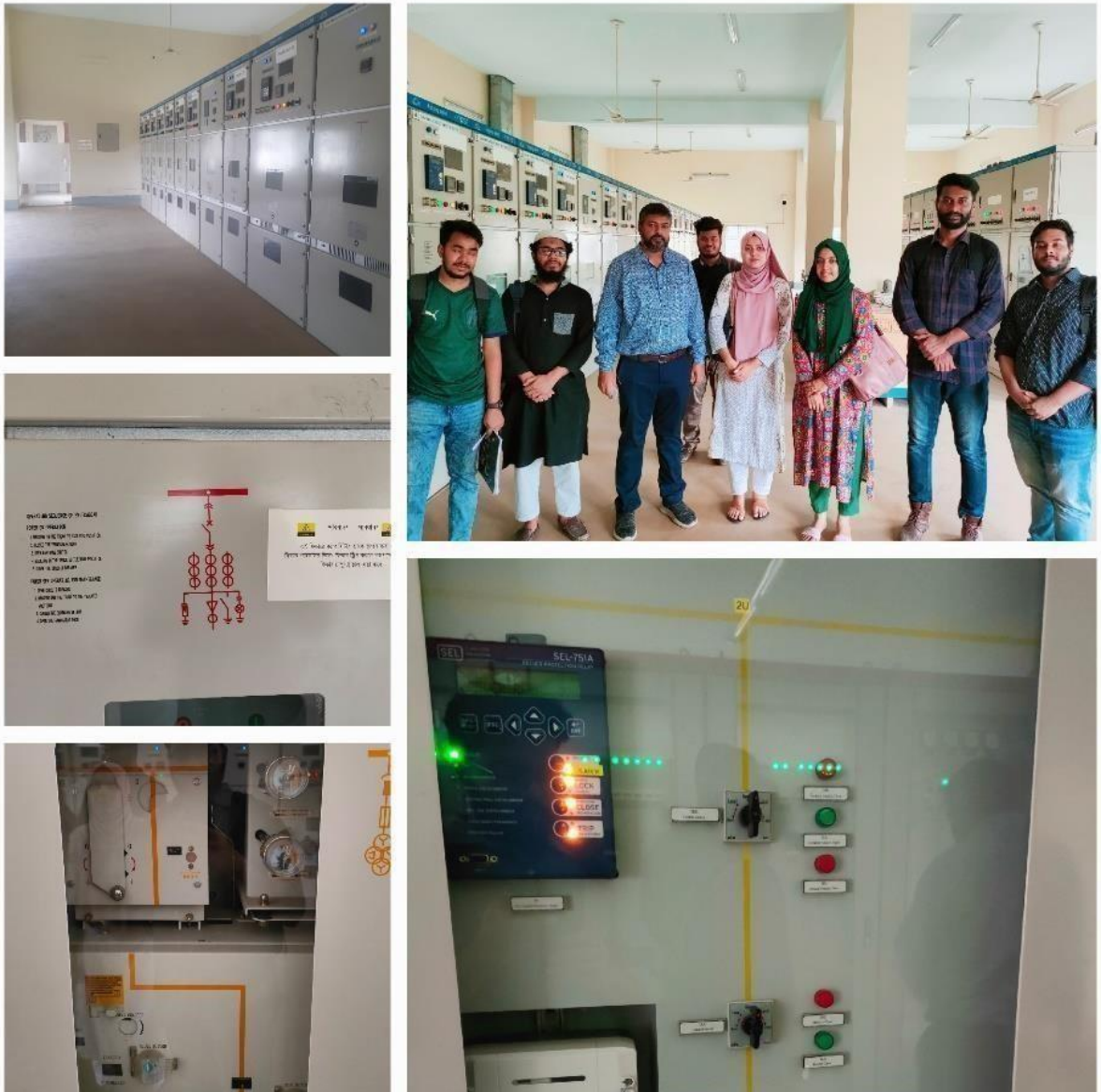
Figure-Grid Sub-Station (Shahjahanpur)
