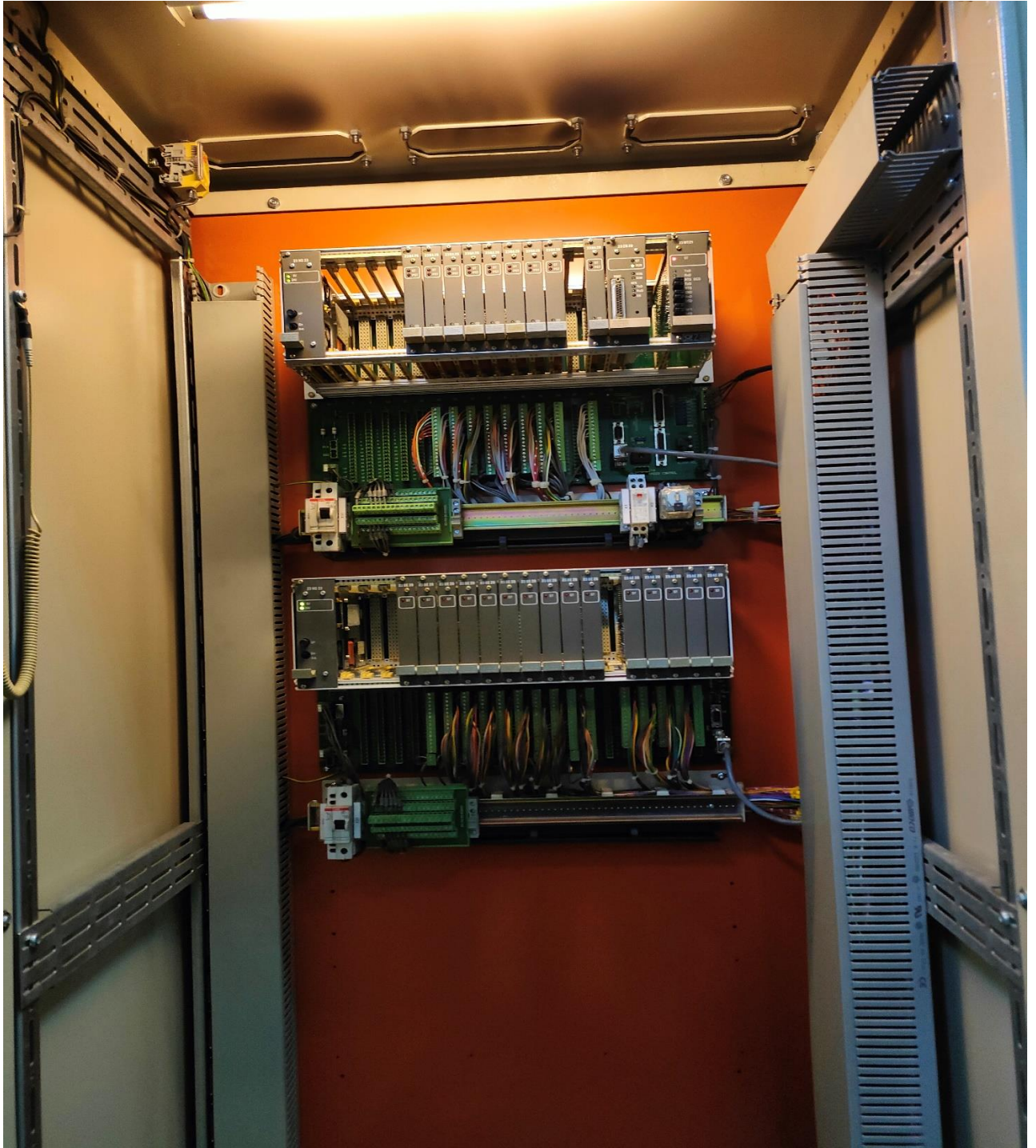
Figure-2: Remote Terminal Unit (RTU)
