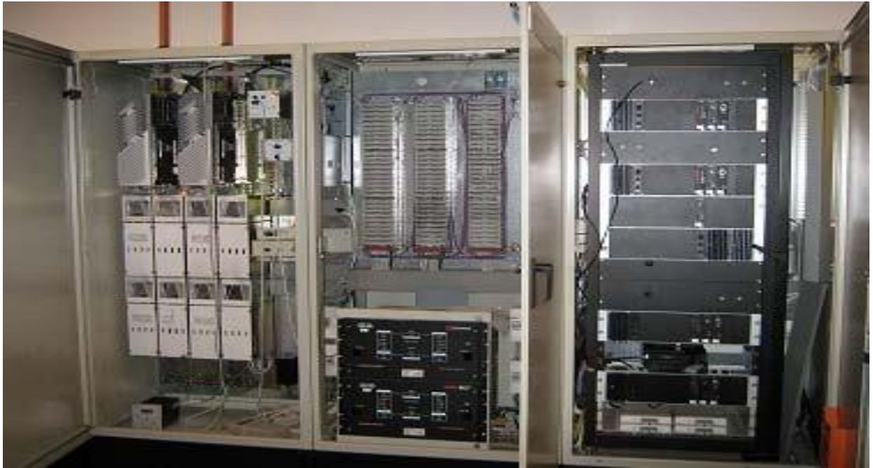
Figure-3: Communication Equipment
