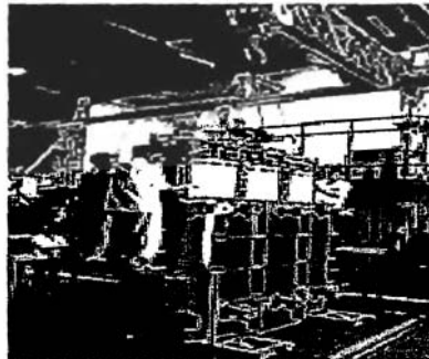
Figure 5:Transformer Tanking up
