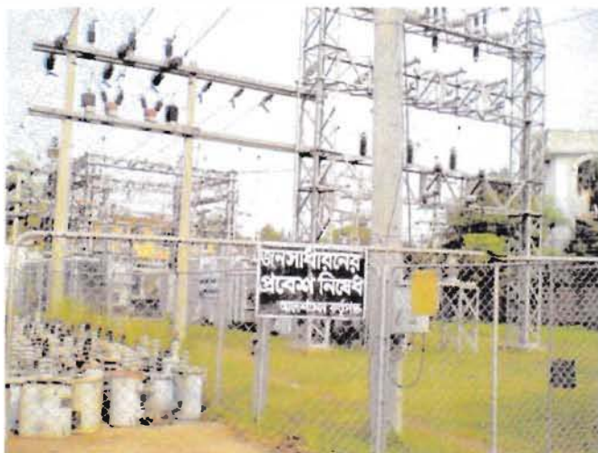
Figure 18: Overall View of the Distribution Substation
