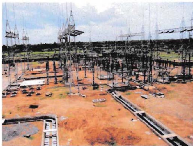
Figure 12: Typical view of a Grid Substation
