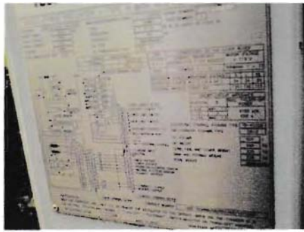
Figure 20: Nameplate of the Transformer
