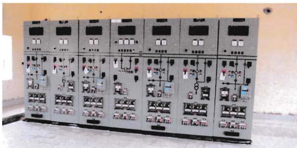
Figure 8: Programmable Logic Control Unit at UPGD
