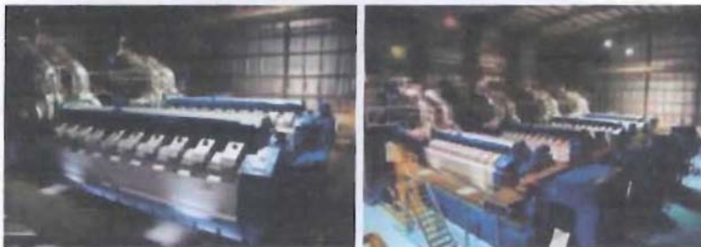
Figure: 4.2: Views of engine room
