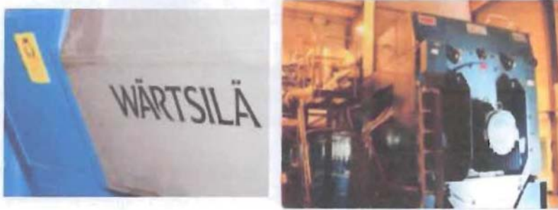
Figure 4.2: Views of engine room
