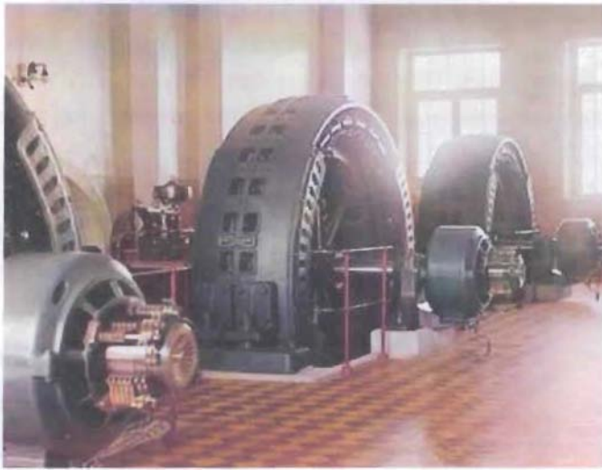
Figure 4.5: Alternator of UPGD power plant
