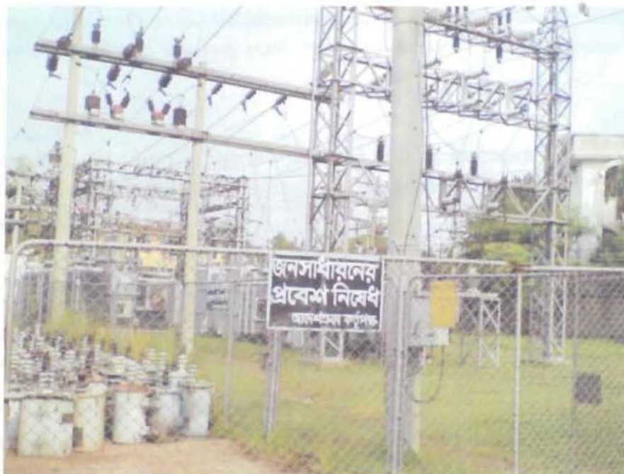
Figure 3.1: Distribution substation of PBS-1
