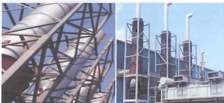
Figure 4.6: Radiators in UPGD power plant
