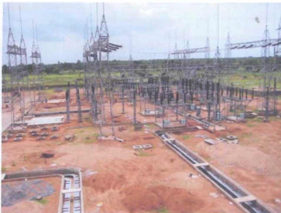
Figure 3.2: View of Grid Substation, Hamannogor, Savar
