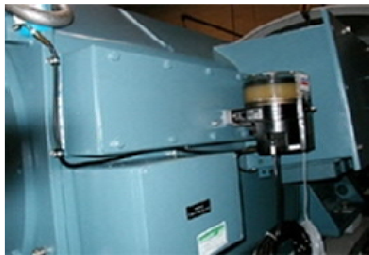
Figure 3.4: Lube Oil pump in the generator of steam turbine [11].
