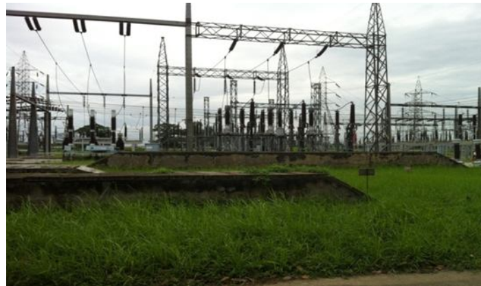
Figure 4.1: Part of a substation of APSCL [11].
