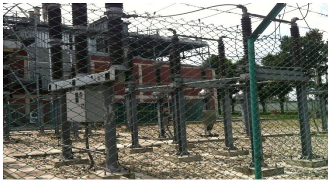
Figure 4.10: Cover of stones in switchyard [11].
