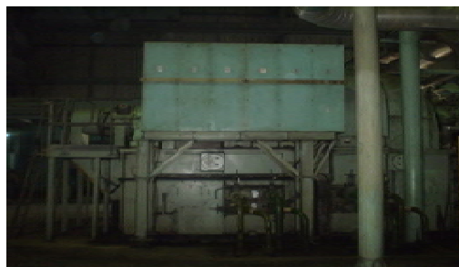
Figure 2.4: Generator to Generate Electricity by Ignited Gas [11].
