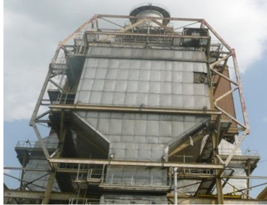
Figure 3.2: A boiler of APSCL [11].
