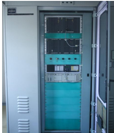
Figure 7.5: Automatic Voltage Regulator
