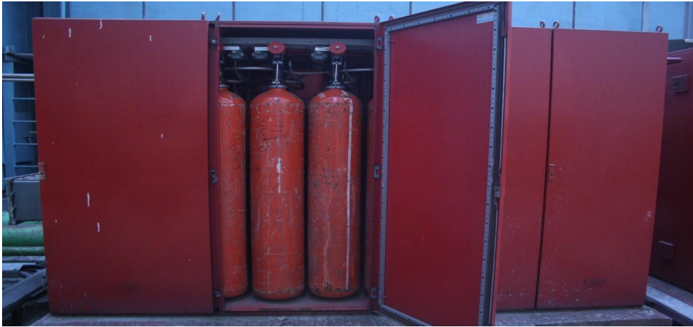
Figure 4.1: CO 2 fire safety cylinders for internal instrument protection in EGCB
