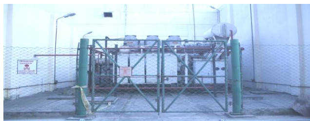
Figure 6.3: Power Transformer-2 of EGCB
