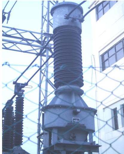
Figure 6.5: Current Transformer of EGCB
