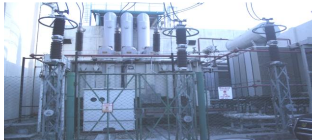
Figure 6.2: Power Transformer-1 of EGCB
