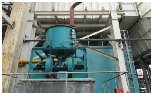
Figure 5.2: Mist Eliminator Pump of EGCB
