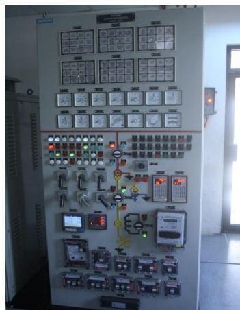
Figure 7.4: Generator Control Panel
