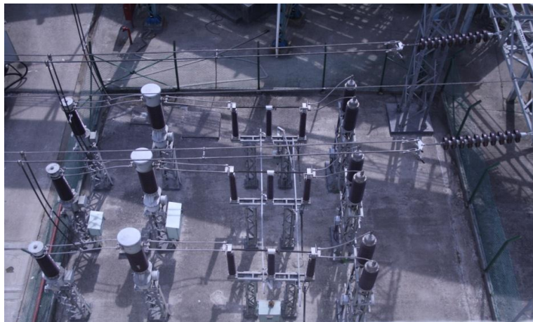
Figure 6.1: The Substation of EGCB
