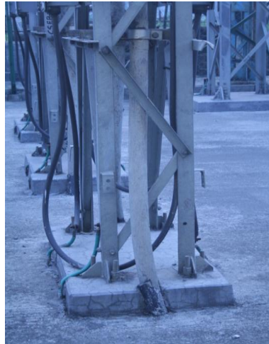
Figure 6.8: Underground Cables of EGCB substation
