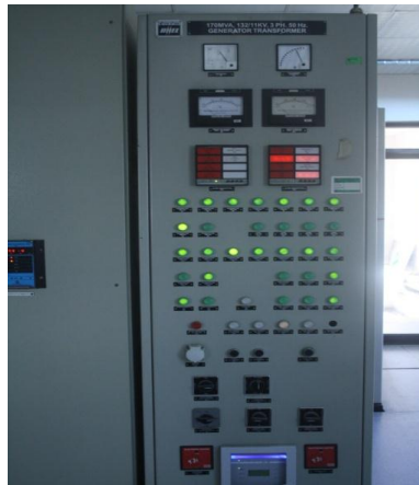
Figure 7.1: Generator Transformer panel
