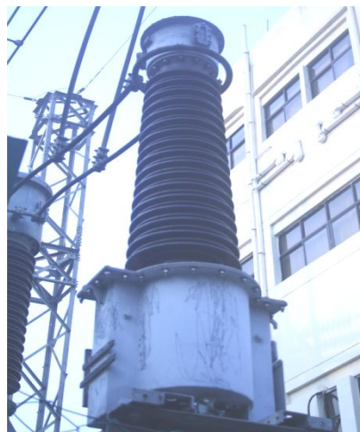
Figure 6.6: Potential Transformers of EGCB
