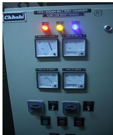
Figure 7.6: Battery Charger Panel
