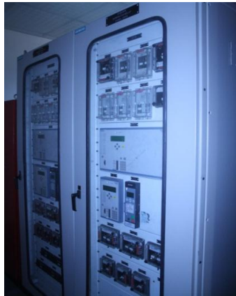
Figure 7.3: Generator Relay Panel
