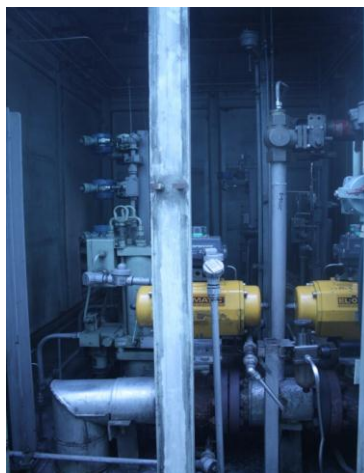
Figure 3.4: Gas Valve Unit of EGCB
