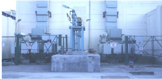
Figure 6.4: Power Transformer 3 and 4 of EGCB
