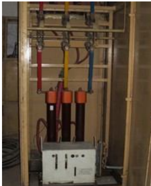
Figure 9.1: High Tension Panel [2].
