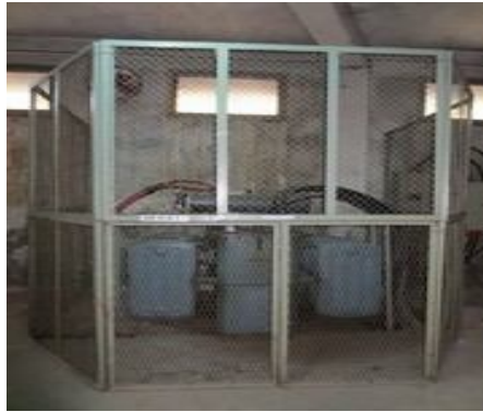
Figure 9.2: Step down Transformer [2].
