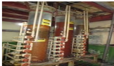
Figure 6.7: DM Water Plant [2].
