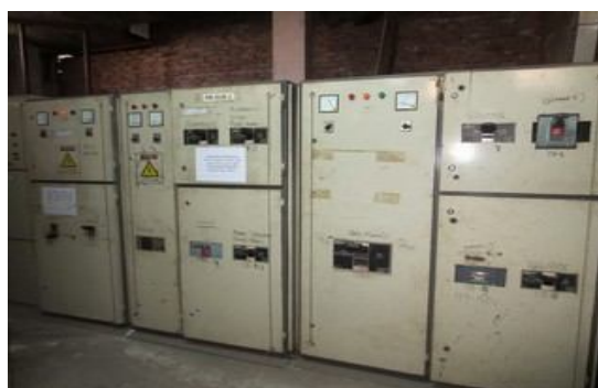
Figure 9.7: Low Tension Panel [2].
