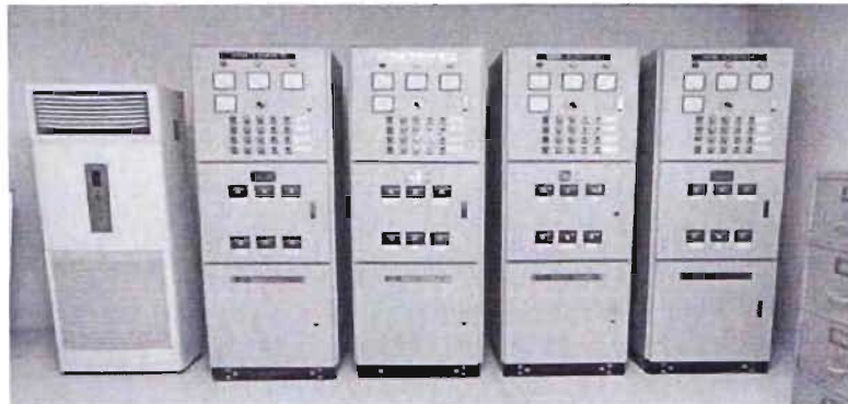
Fig 5.1: LT switchgear panel
