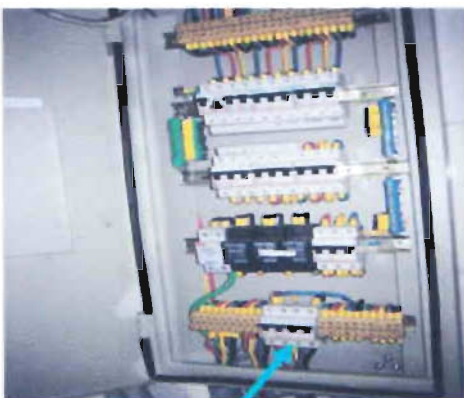
Main Circuit Breaker (MCB)
