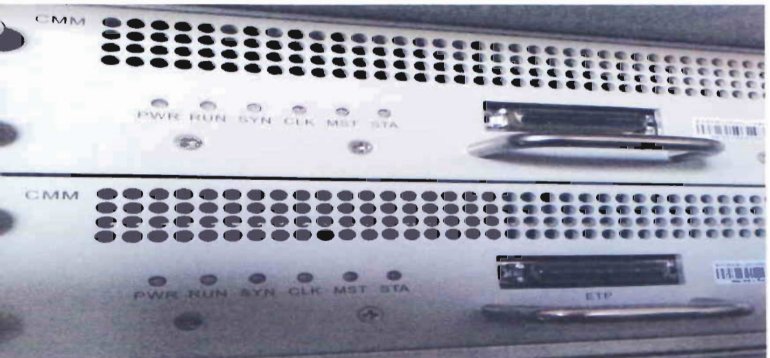
Figure 4.15: Controller & Maintenance Module (CMM) Alarm
