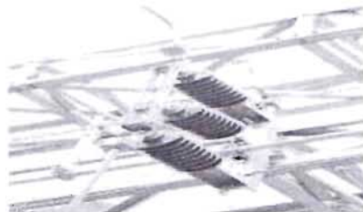
Figure 16: Centre Break Isolator
