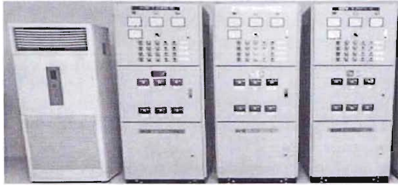
Figure 5: LT switchgear panel
