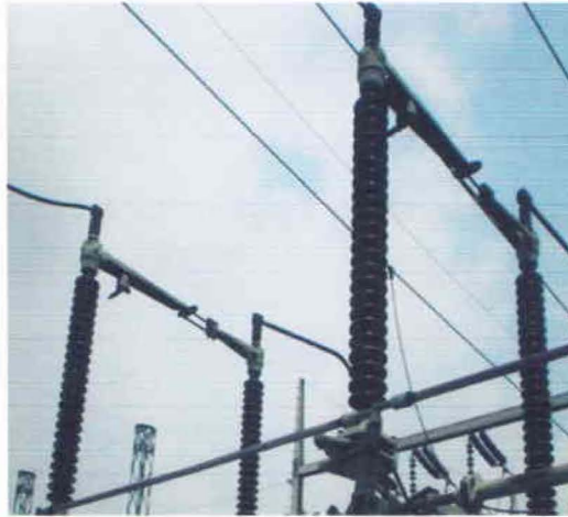
Figure 4.11: Isolators used in APSCL (Rated voltage 252KV, rated current maximum 2500 A)
