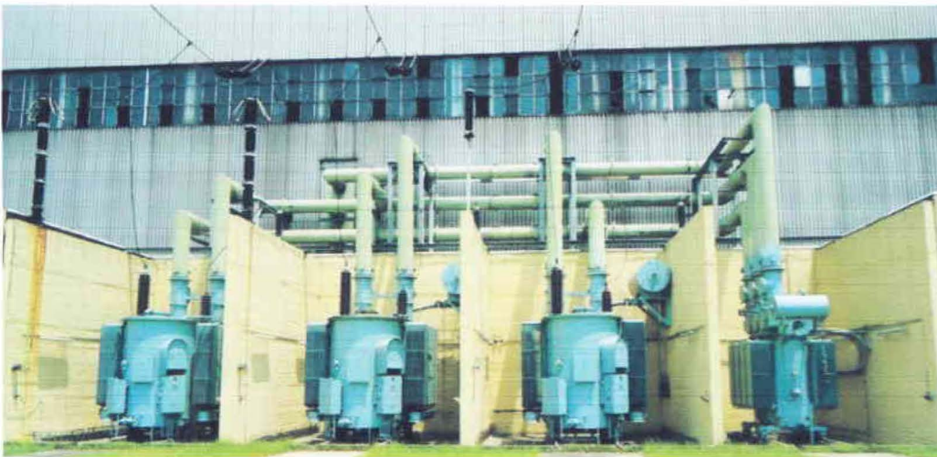
Figure 4.12: Wye to delta conversion (3-single phase and a three phase transformer) and transmission
