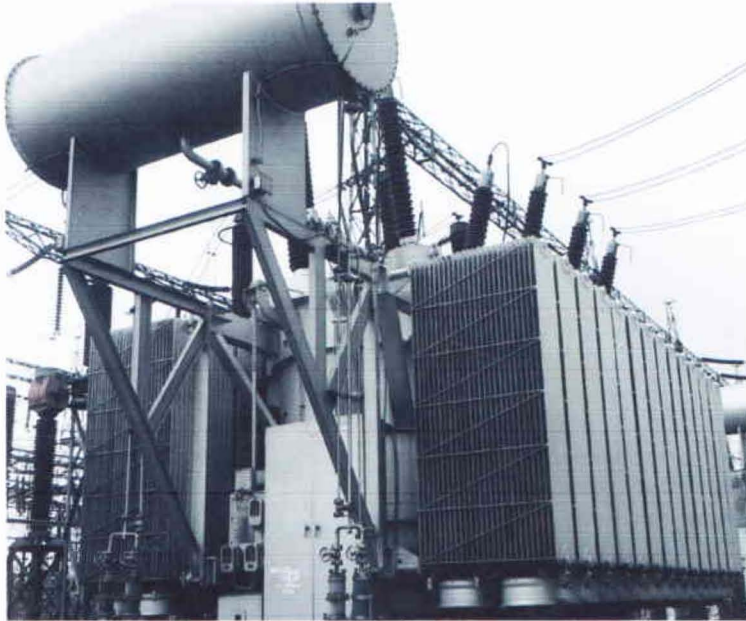
Figure 4.1: A Step up Power Transformer of APSCL
