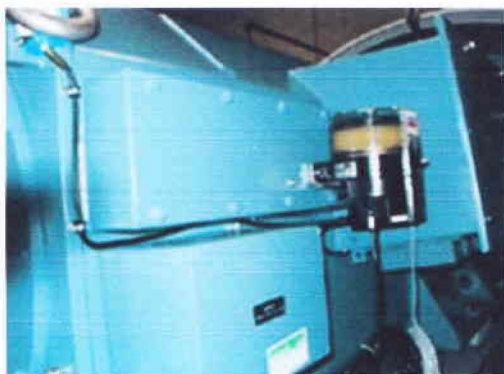
Figure 2.3: Lube Oil pump in the generator of steam turbine
