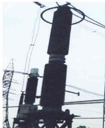
Figure 4.14: Lightning Arrester arrangement in the substation
