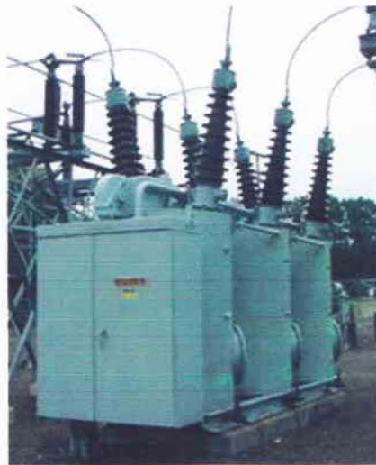
Figure 4.8: Oil Circuit Breaker in substation rated voltage of 132 KV and Current 1250 A
