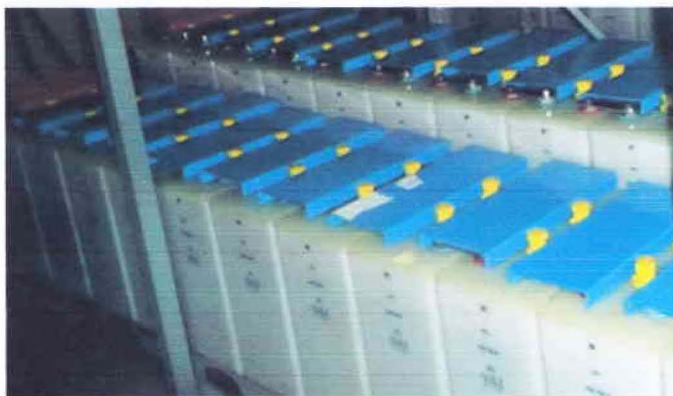
Figure 4.19: Series Connection of NiCd battery in battery backup room
