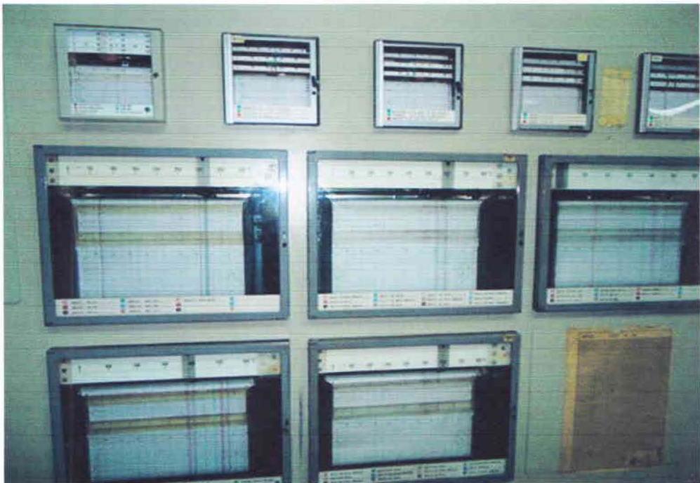
Figure 4.16: Data (frequency, speed, temperature, current, voltage) record in graphical form in unit 1 and 2 control room
