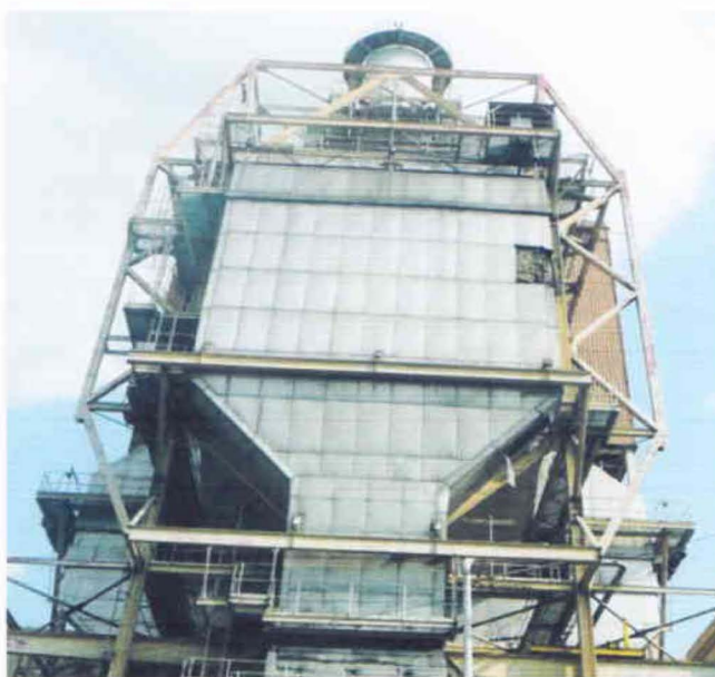
Figure 2.2: A boiler of APSCL in steam turbine
