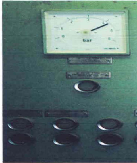
Figure 2.4: Pressure measurement and control panel beside the generator
