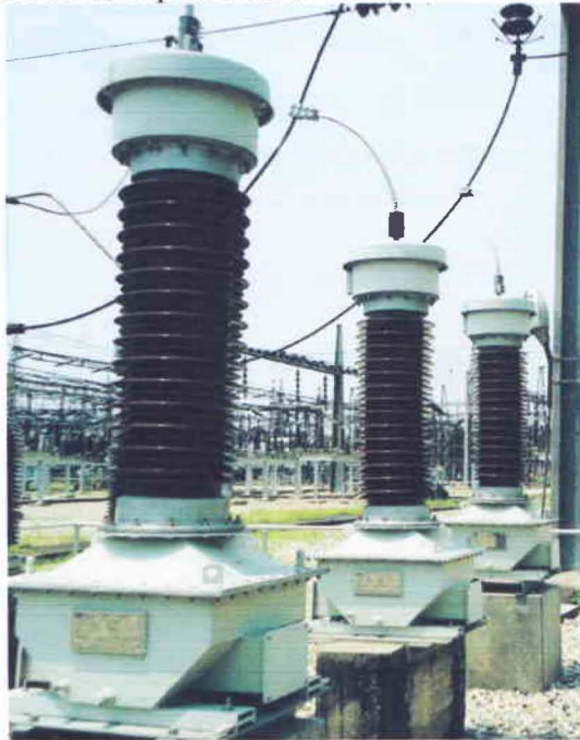
Figure 4.4: Single Phase, 132 KV outdoor Potential Transformer of APSCL
