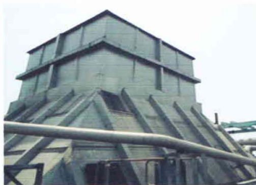
Figure 3.5: Chimney of Waste heat recovery unit in combined cycle plant
