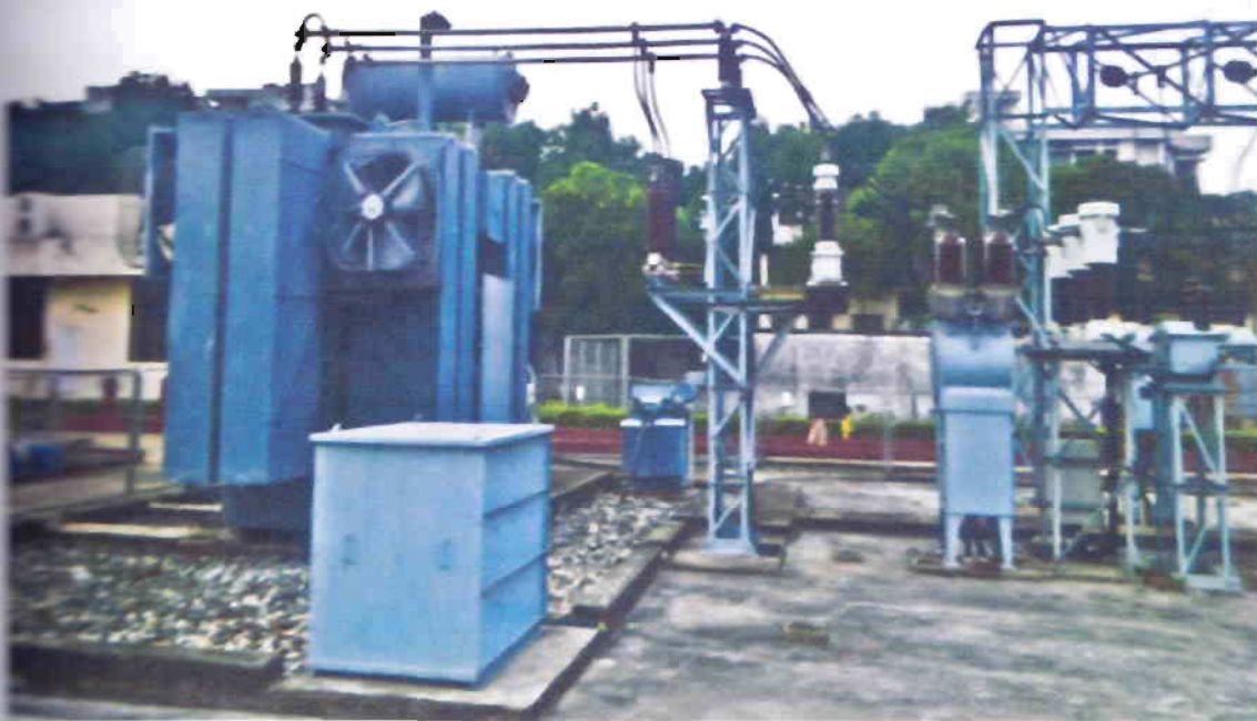
Figure 2.4: 132/33KV transformer in Digun grid substation.
