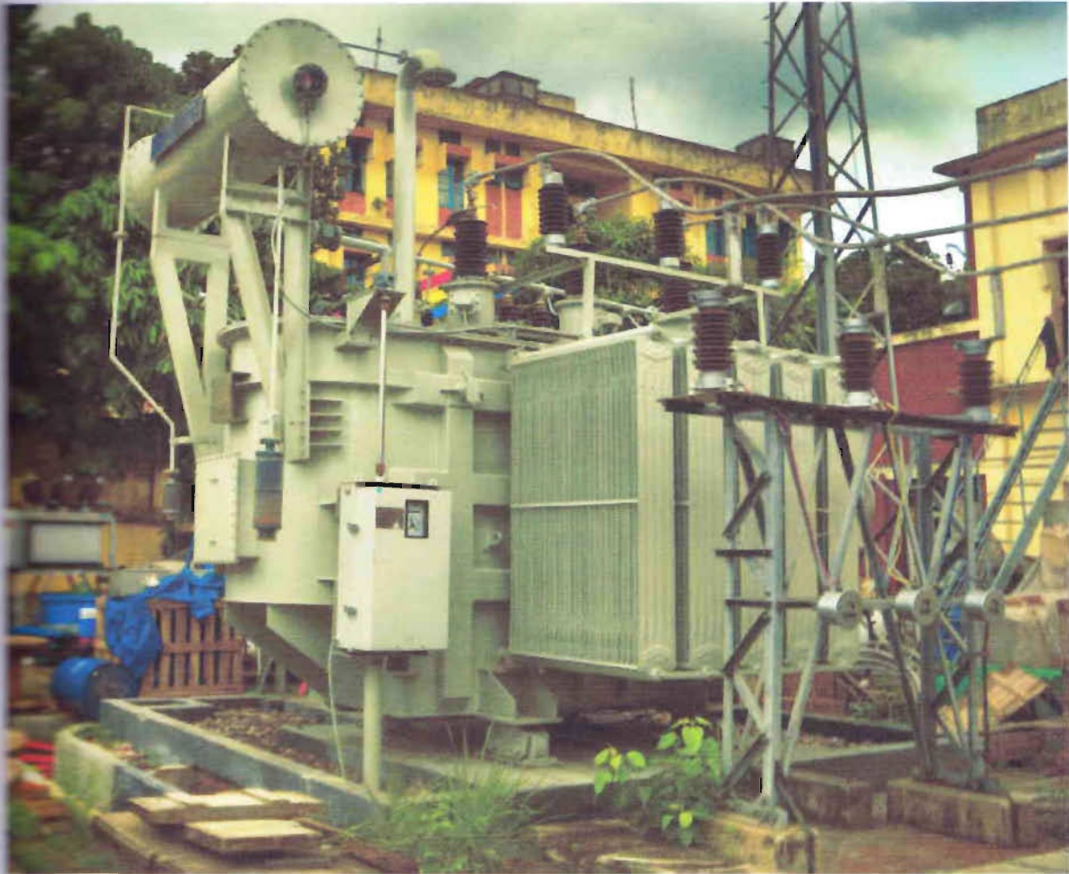
Figure 2.3: Power Transformer in Kafrul substation
