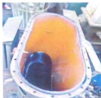
Figure 3.7: Opened transformer tank and burnt oil.
