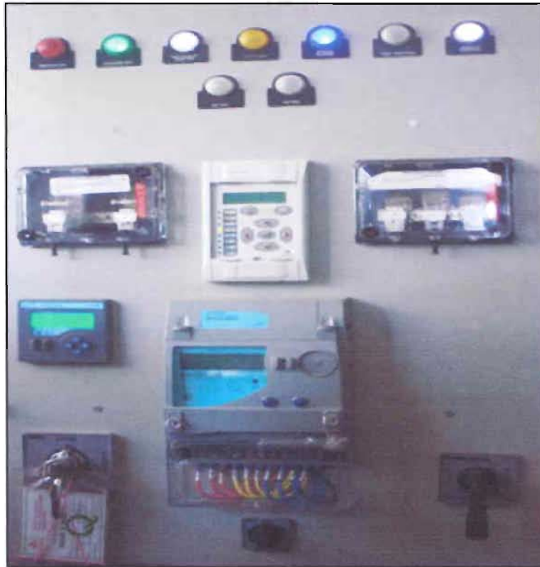
Figure 2.15: Control panel (Kafrul Control Panel)
