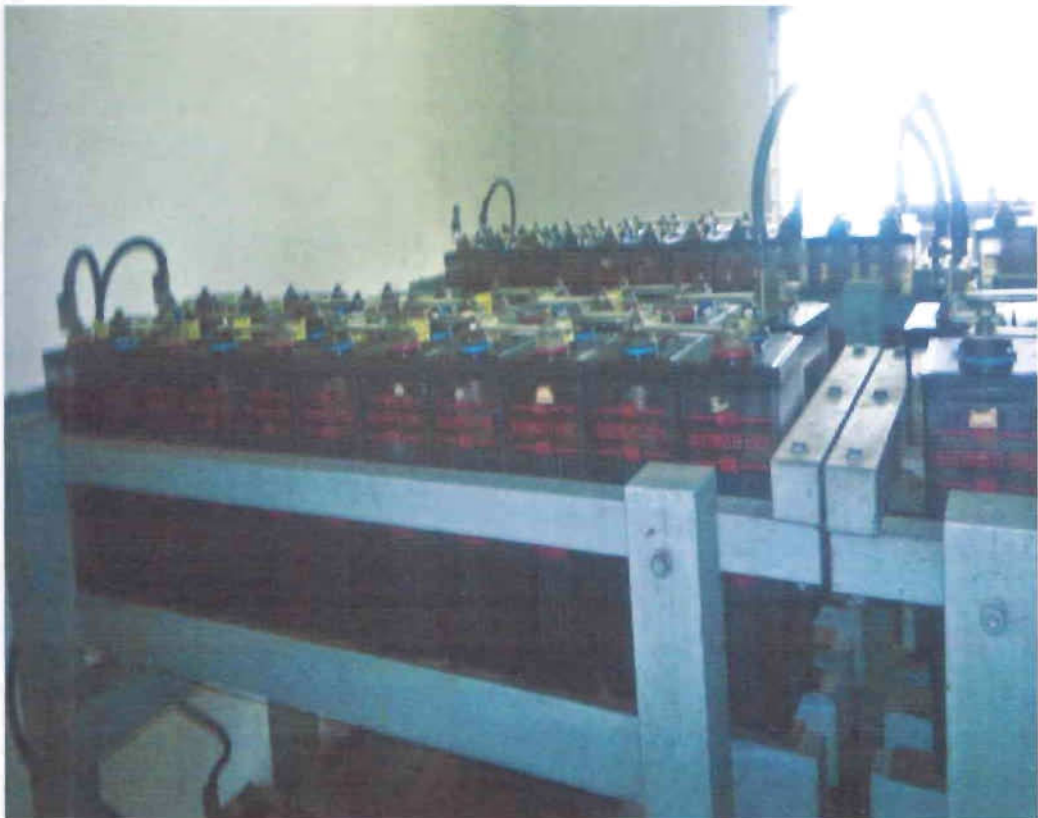
Figure 2.12: Backup battery section of Kafrul 33/11KV substation.
