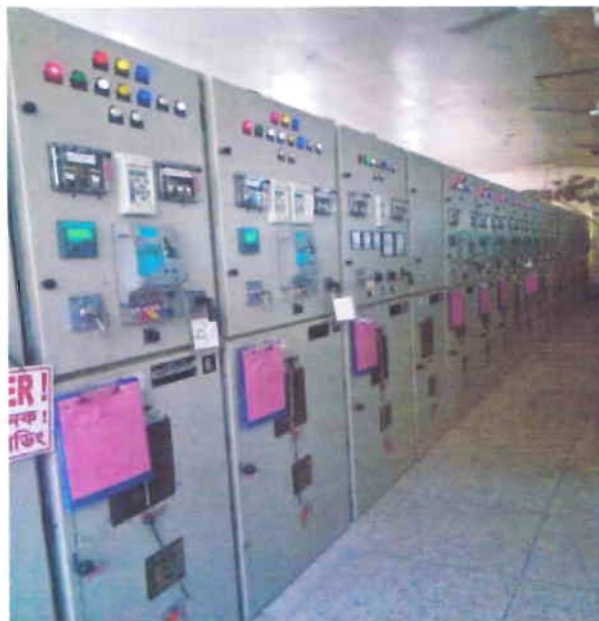
Figure 2.17: Control room of Kafrul 33/11KV substation.
