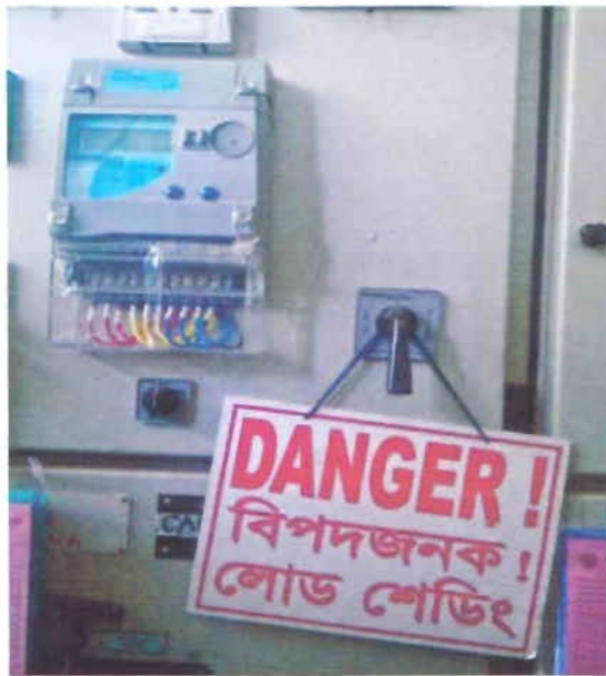
Figure 2.18: Danger sign to remind operator that breaker is on or load shading going on.
