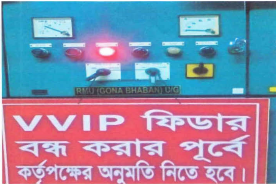
Figure 2.20: VVIP feeder's control panel of Prime Minister's home
