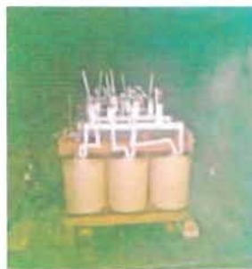
Figure 3.9: Dark chamber where inside body of transformer heated up to 70 degree Celsius.
