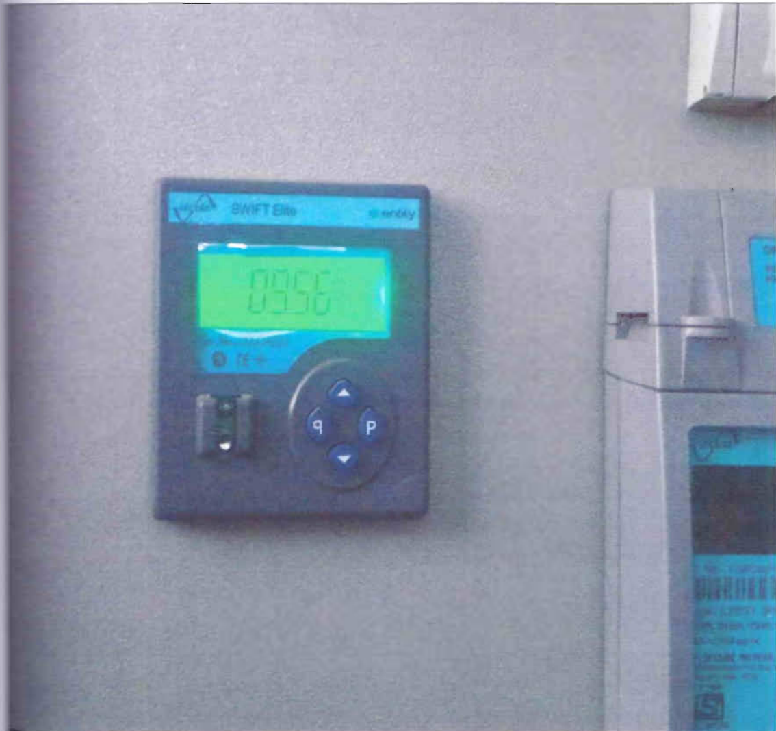
Figure 2.19: Power factor monitor display in control panel.
