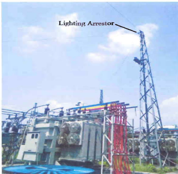
Figure 7.11: Lighting Arrestors in Mirpur-14 Substation
