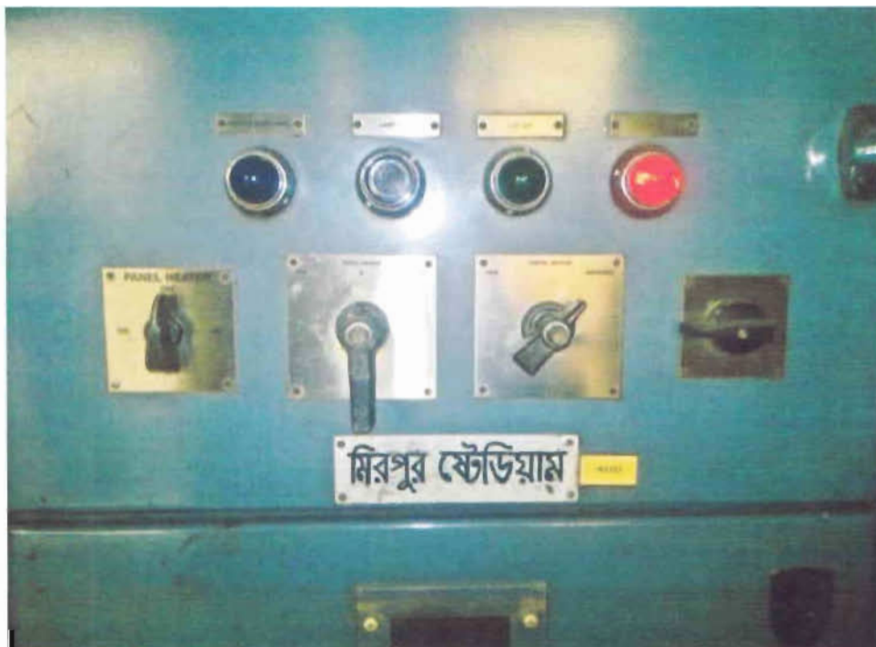
Figure 2.21: Control panel of Mirpur National Cricket Stadium.
