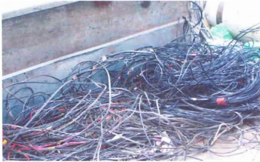
Figure 5.1 : Disconnection of illegal connection
