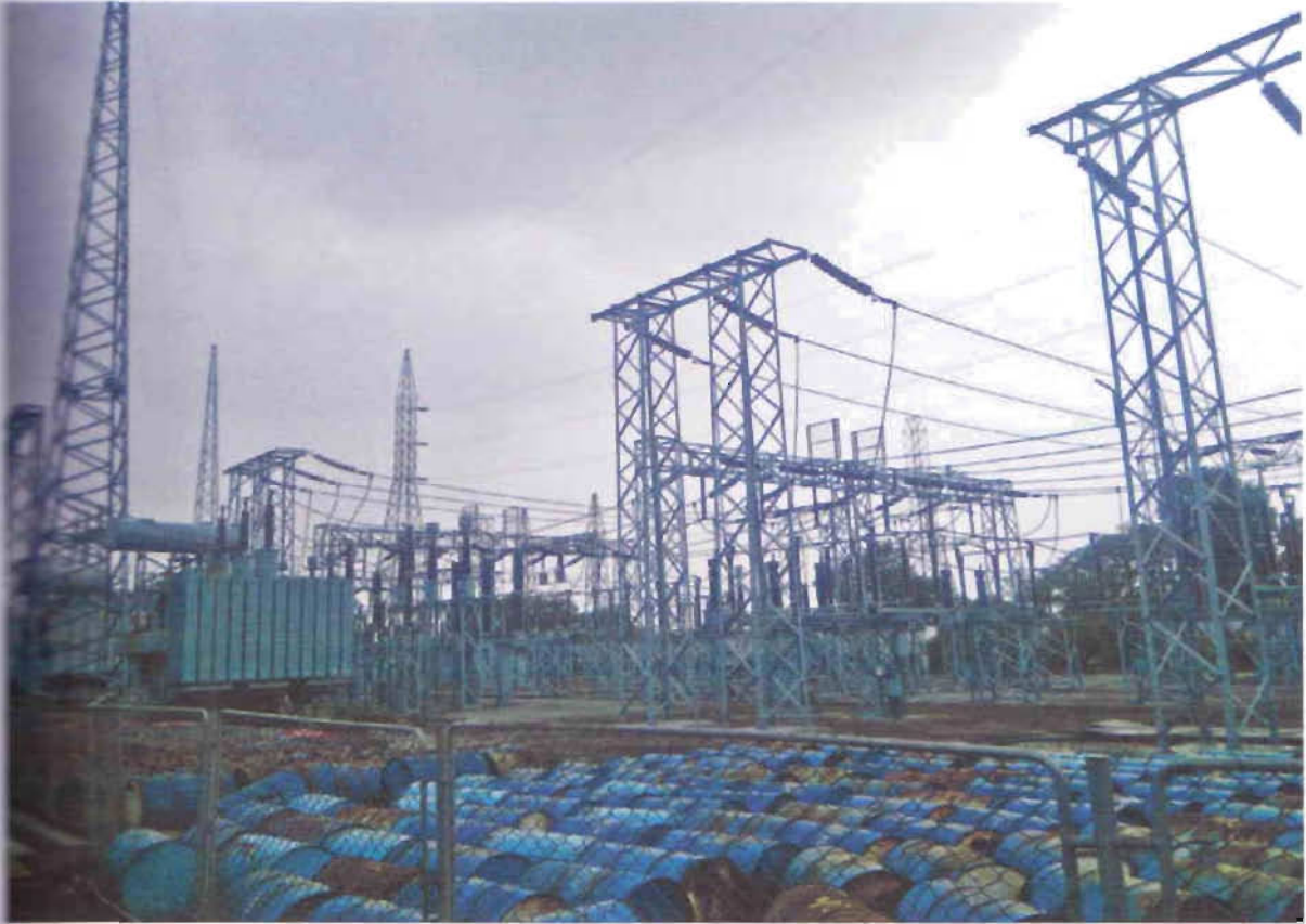
Fig: 2.2 Grid substation of Kallyanpur grid (Digun grid)
