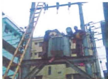
Figure 4.13: Connection was given to H.T line. to the H.T side of transformer.
