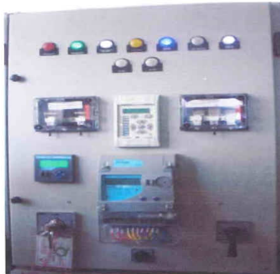
Fig 2.16: A substation control room switching unit
