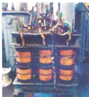
Figure 3.8: Opened Core and Coils of transformer.
