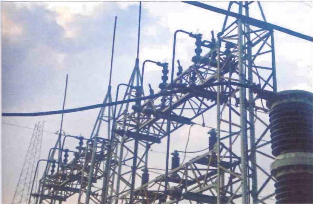
Figure 2.10 Bus bar system in Digun 132/33KV grid substation.
