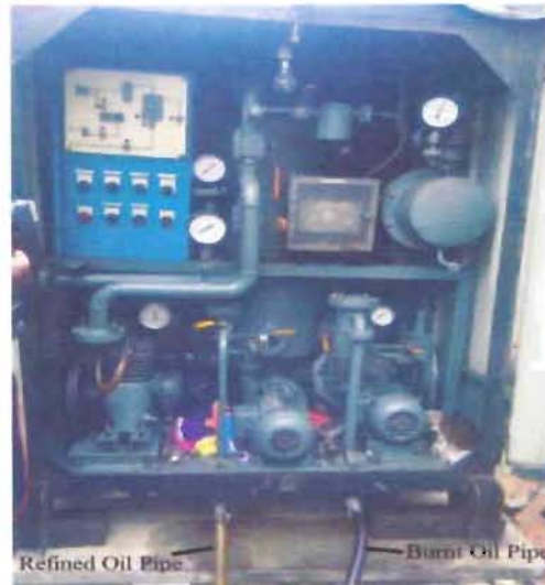
Figure 3.10:1000 LPH oil filtration plant
