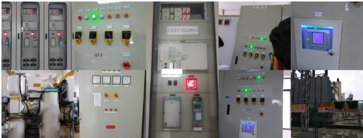
Figure-18: Dhanmondi Substation Visit
