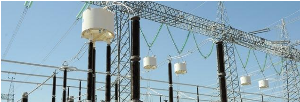
Figure-11: Line Trap Unit in Substation
