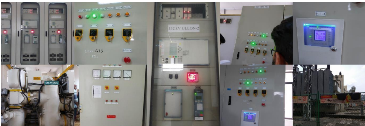
Figure-18: Dhanmondi Substation (2)
