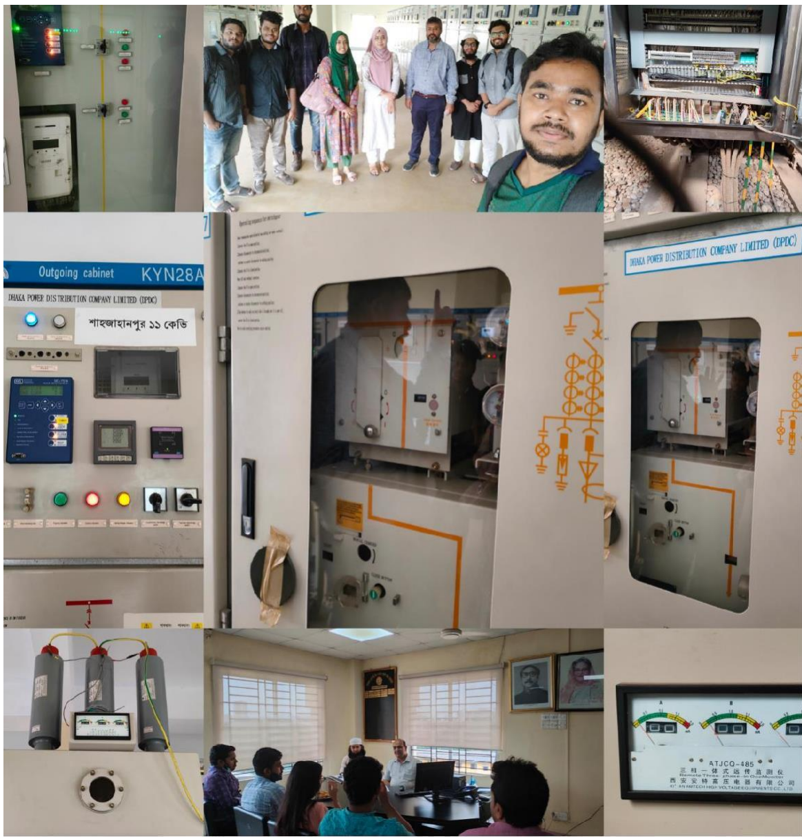
Figure-19: Grid Sub-station Visit
