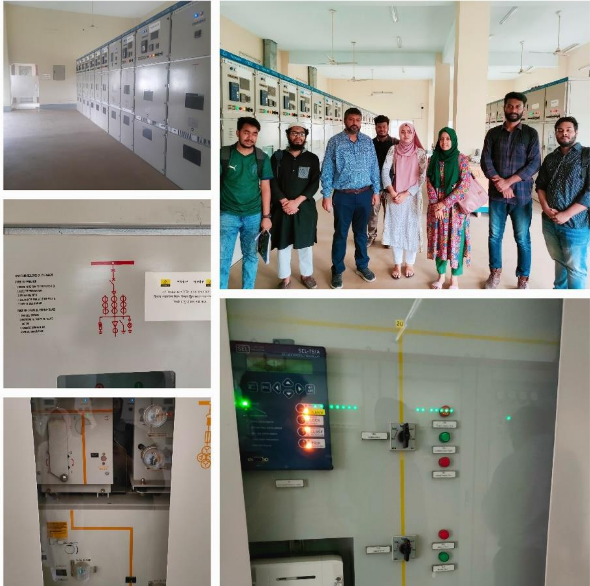
Figure 13: Grid Sub-Station (Shahjahanpur)
