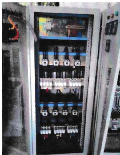
Figure 33: PFI (power factor improver)
