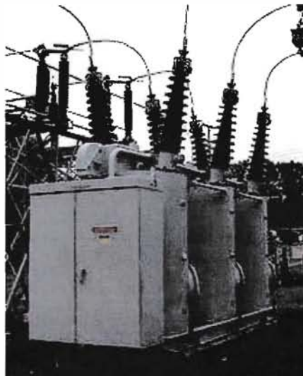
Figure11: 400 kV SF 6 live tank circuit breakers
