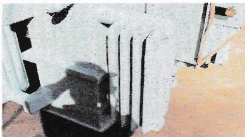
Figure 12: Cooling system of Transformer
