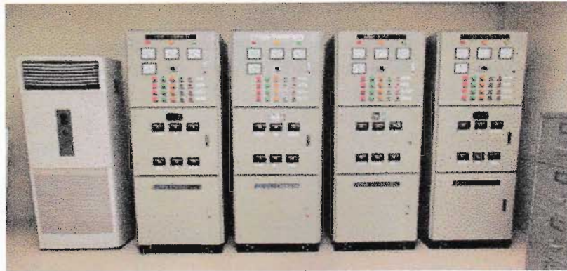
Figure 19: LT switchgear panel
