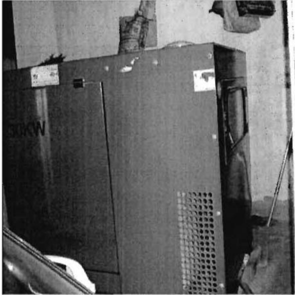
Figure 19: The Generator Box
