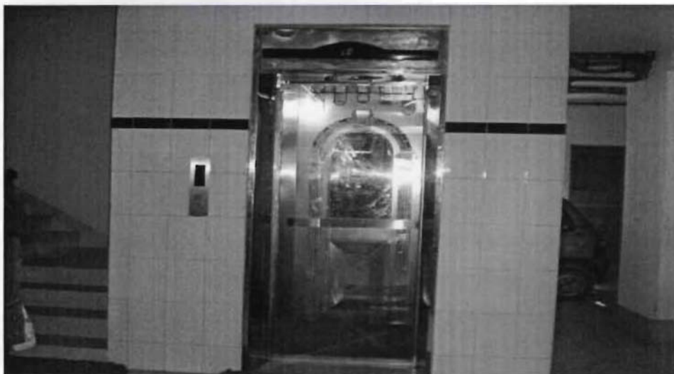
Figure 1: The Lift Cabin
