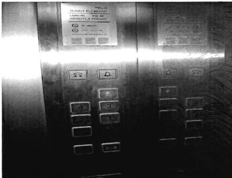
Figure 4: The Switch Board inside the Lift Cabin
