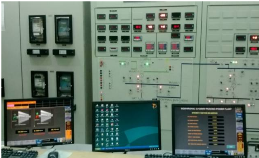
Figure 6.1: Main control room [2]
