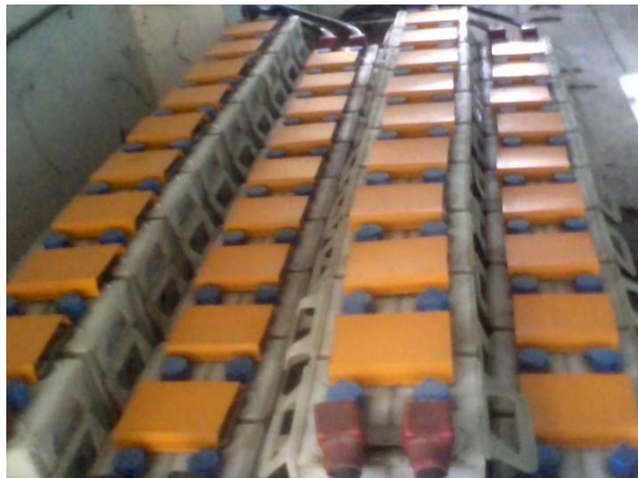
Figure 9.1: Auxiliary DC power supply [2]
