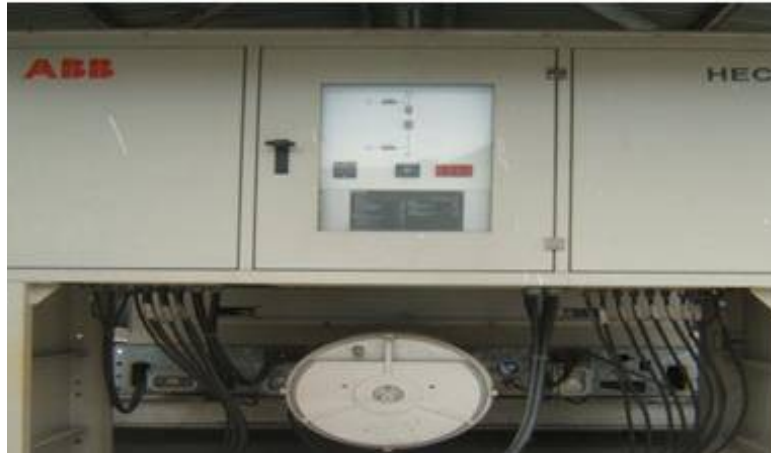
Figure 5.2: SF 6 circuit breaker [2]
