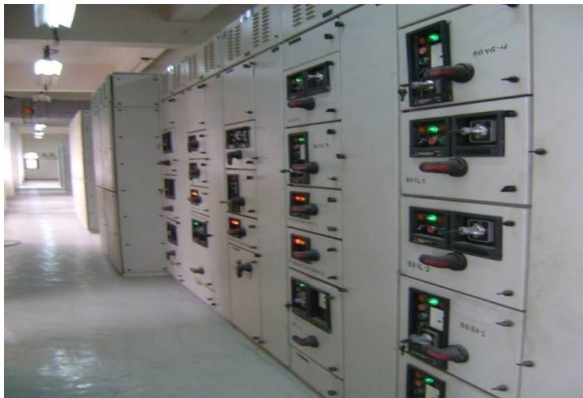
Figure 6.3: One side view of manual control room [2]
