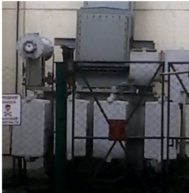
Figure 3.3: Unit auxiliary transformer [2]
