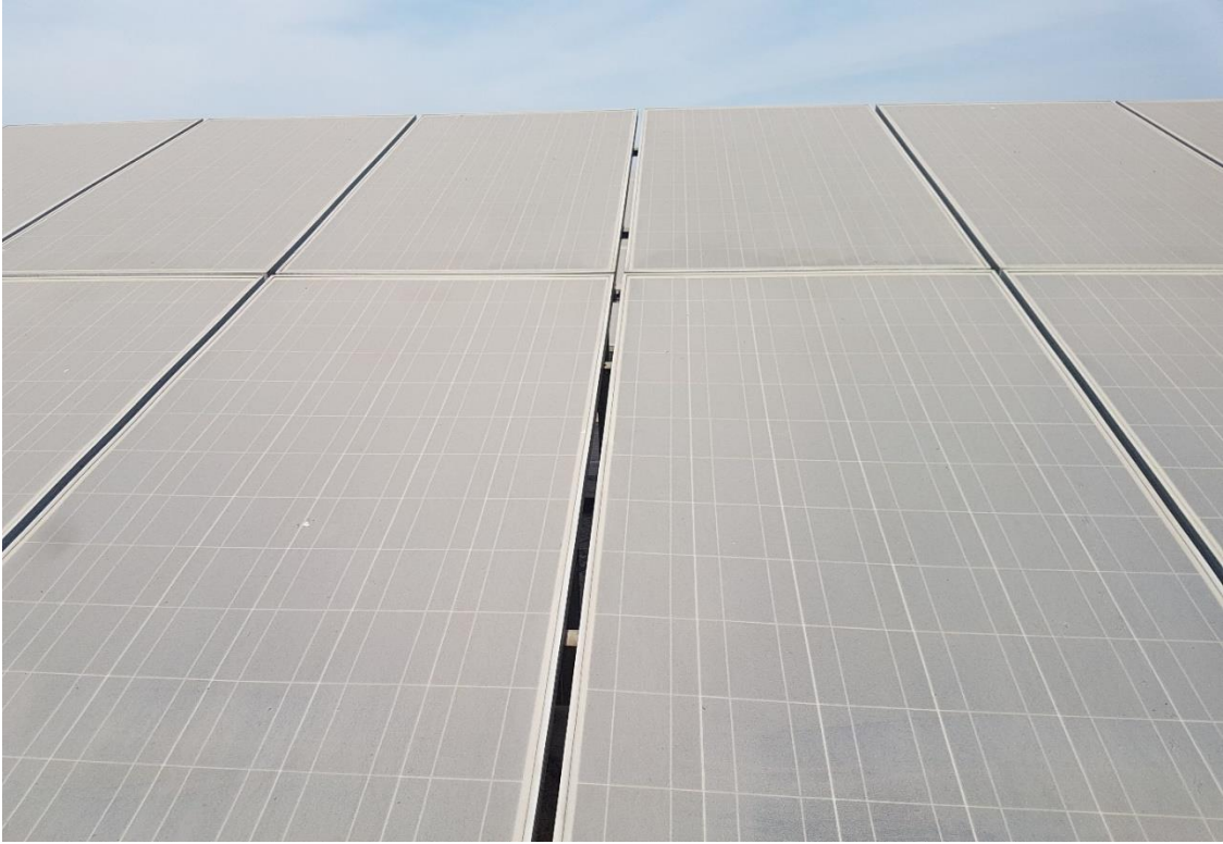
Figure 4.8: PV panels of the system.
